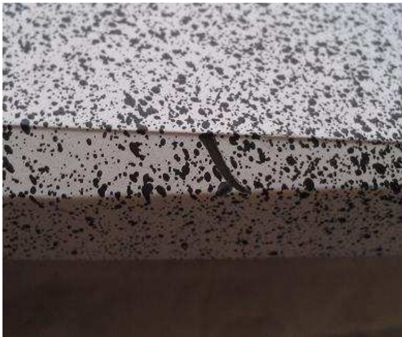
Figure 76: Spec 2 Surf Failure
