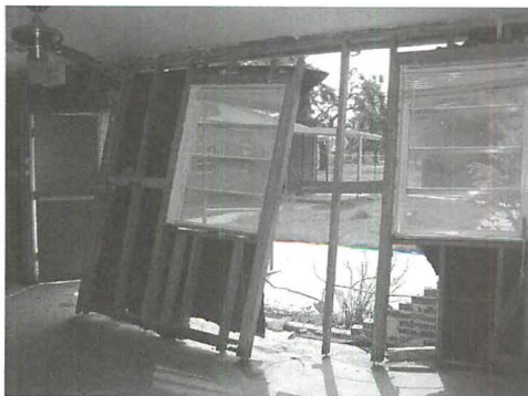
Our Lady of Prompt Succor Elementary School sustained an astonishing level of damage due to Katrina and subsequent flooding. (Photo by Jill McKinstry)
