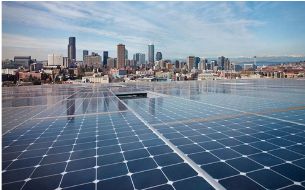
Fig.3. Bullitt Center Roof with 575 BIPV
