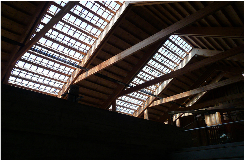
Figure 26. Skylights. Photo courtesy of Peter Cohan.
