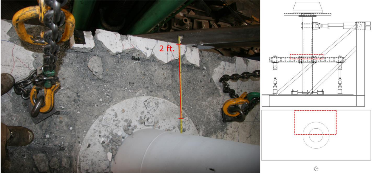
Figure 4-96: Top Joint East Side Crushing – 6.4% Drift (PTB_9_2_0)
