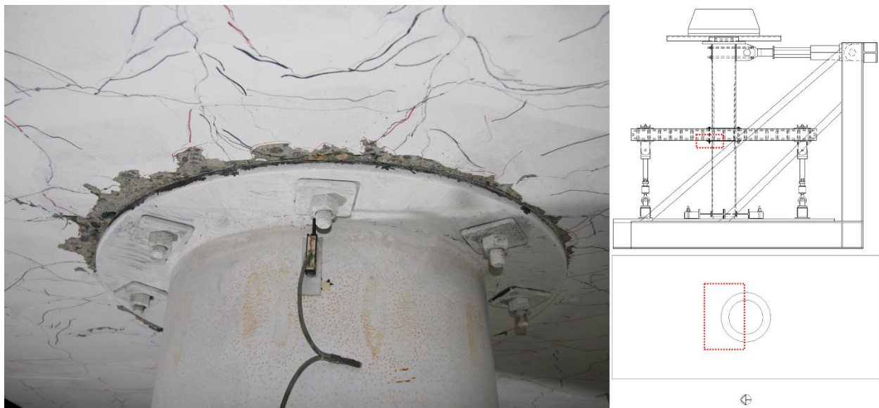
Figure 4-3: Example Spalling around Bottom Joint
