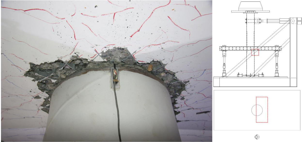
Figure 4-22: Bottom Joint South Side Crushing – 4.2% Drift (SR_4_10_5)
