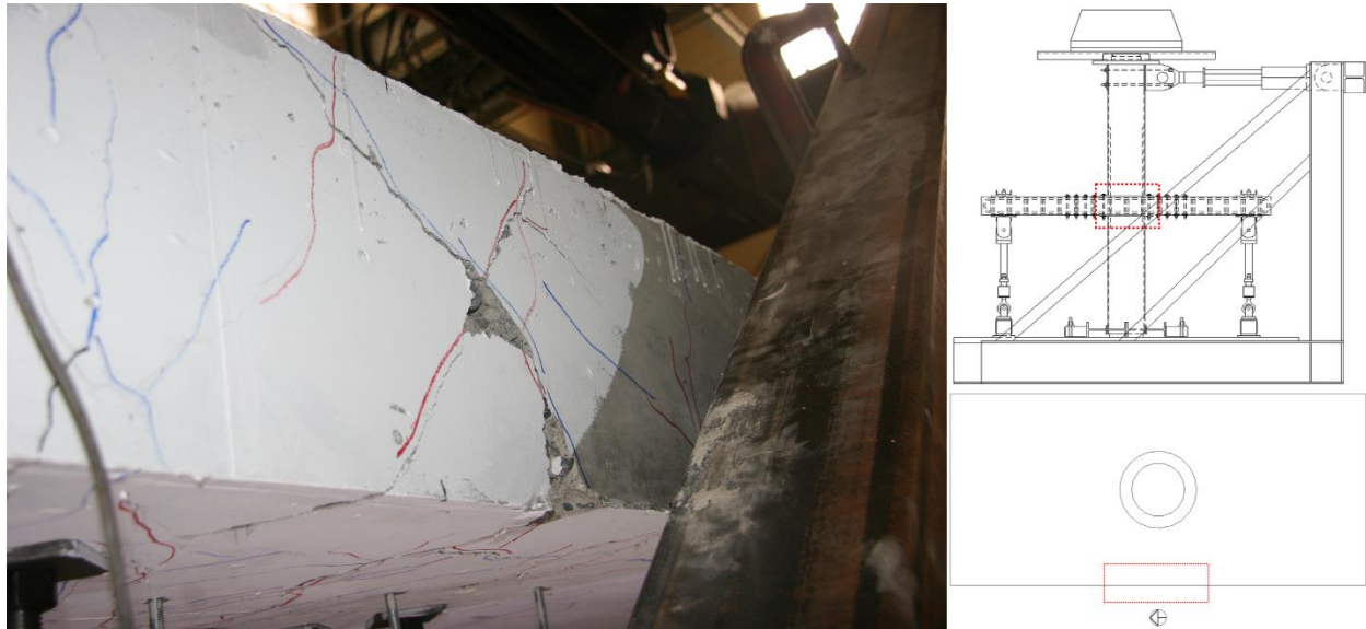
Figure 4-66: West Edge Shear Cracking – 5.5% Drift (PTB_4.5_1_4)
