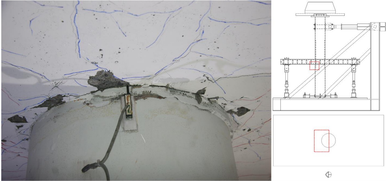
Figure 4-20: Bottom Joint North Side Spalling - 2.8% Drift (SR_4_10_5)
