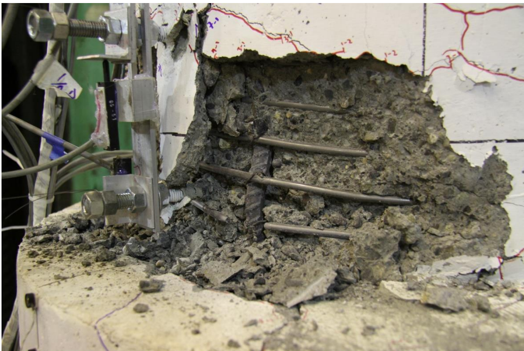
Figure C-0-5. DS-1 – First column spiral fractured at 8.43/--8.27 percent drift
