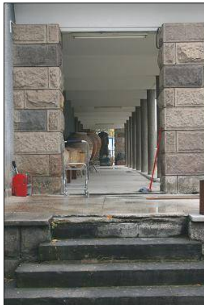
Figure 7.10: Stone covered columns of the portico (From the personal collection of Hikmet Eldek).
