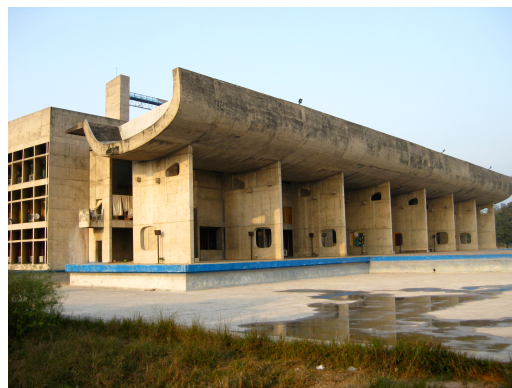
Figure 19: Rehabilitation Needed at the Capitol Complex
