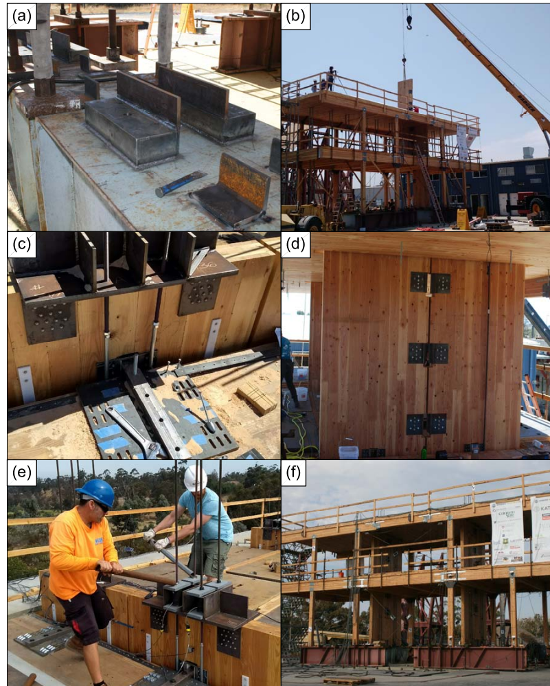
Figure 4.24: Rocking wall construction sequence (a) base beam connections (b) wall installation (c) PT saddle and tongue connection (d) wall without UFPs installed (e) post-tensioning (f) completed specimen
