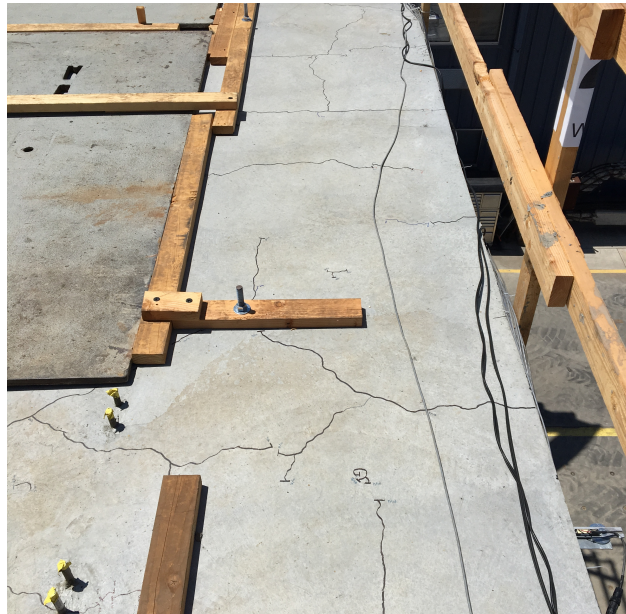
Figure 5.12: Concrete cracking on the roof diaphragm
