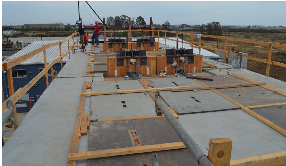
Figure 4.20: Photo of additional seismic mass on the roof held down by the wood grid
