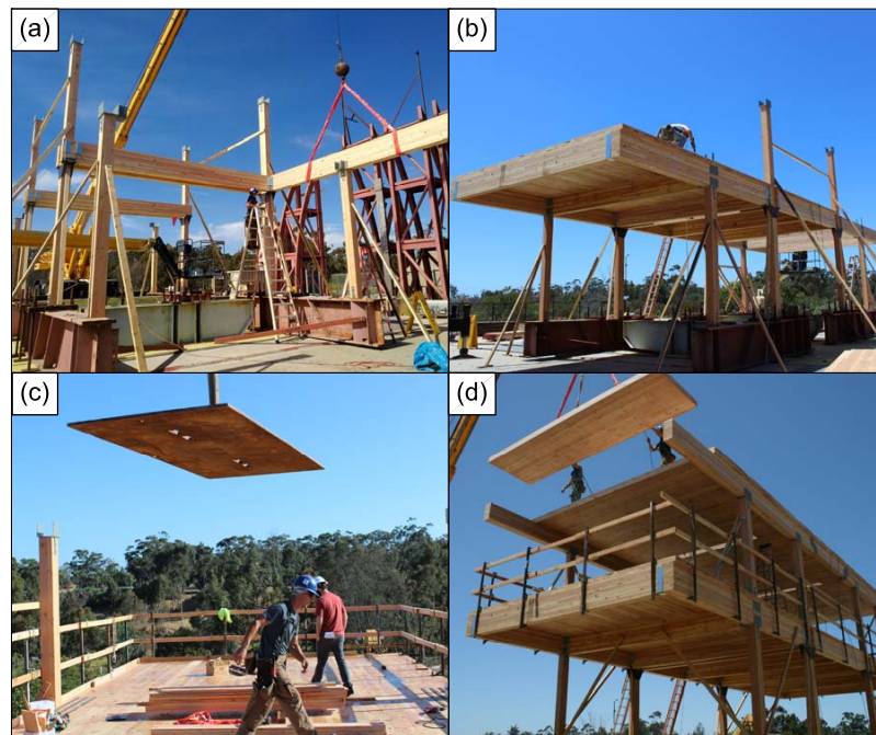
Figure 4.22: Gravity frame construction sequence (a) beam and column gravity frame (b) floor diaphragm panels (c) floor seismic mass (d) roof diaphragm panels
