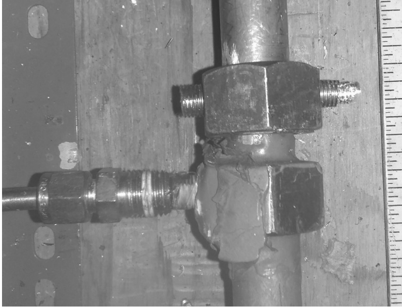
Fig. 11: Shear pin fixture (top) and driven section gas supply line (bottom).
