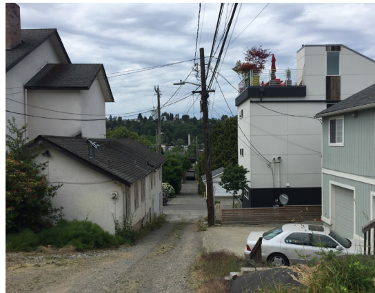
The former Mission Baptist Church, under demolition during this project, is adjacent to new million dollar speculative home development.
