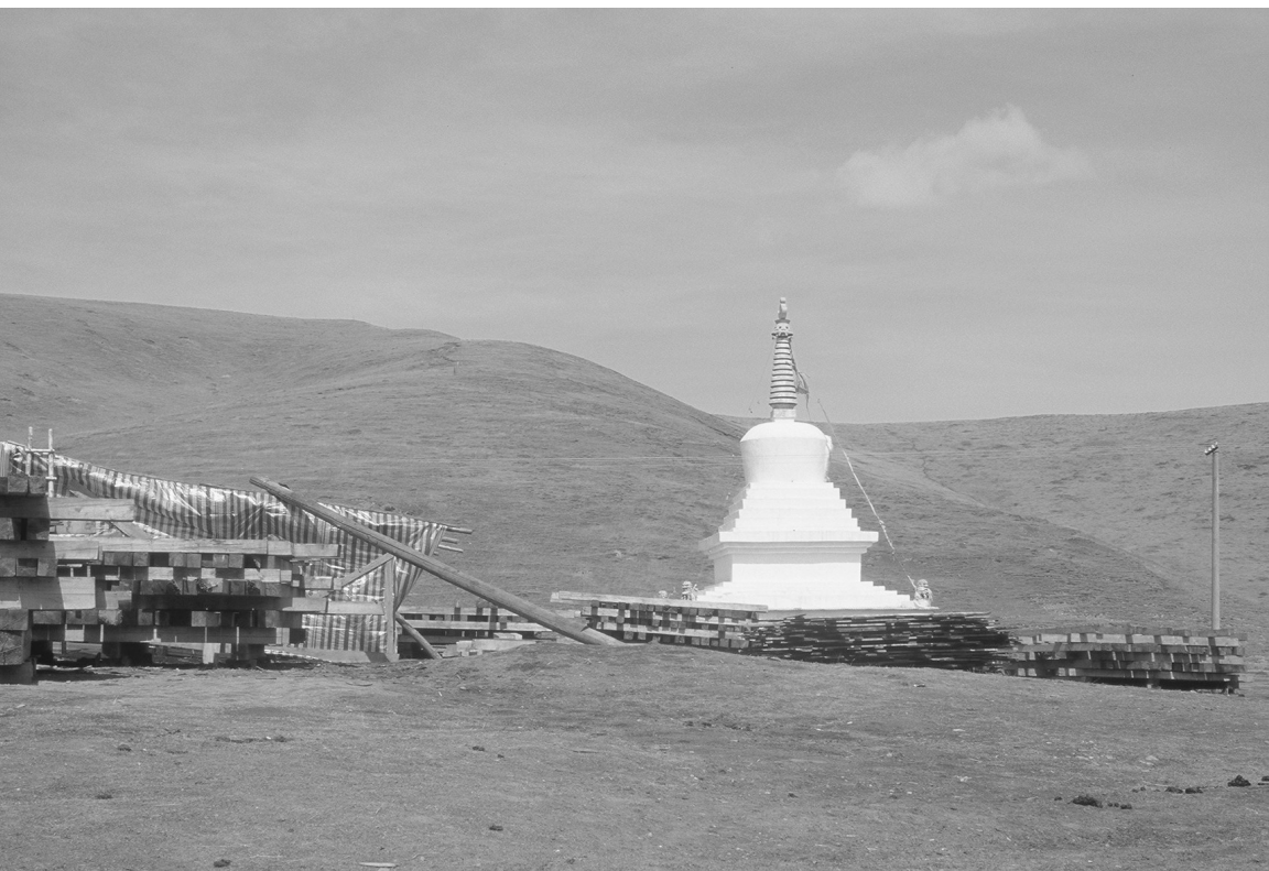
FIG. 2.8. A new stupa under construction at Machu Monastery, Kanlho. The work was performed by Tibetans and Han migrant workers from Qinghai.
