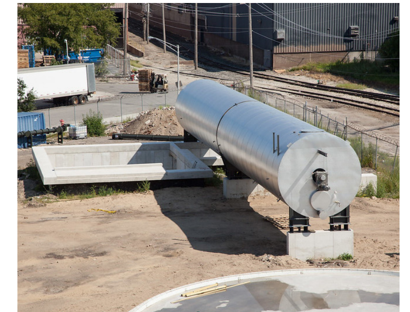
Figure 21: Anaerobic digester installation
