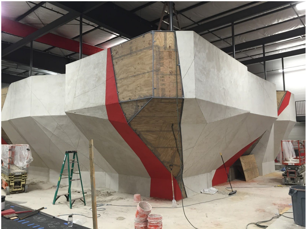
Figure 15: Almost finished climbing wall, with visible slurry, cuts, and sweeping compound being used.
