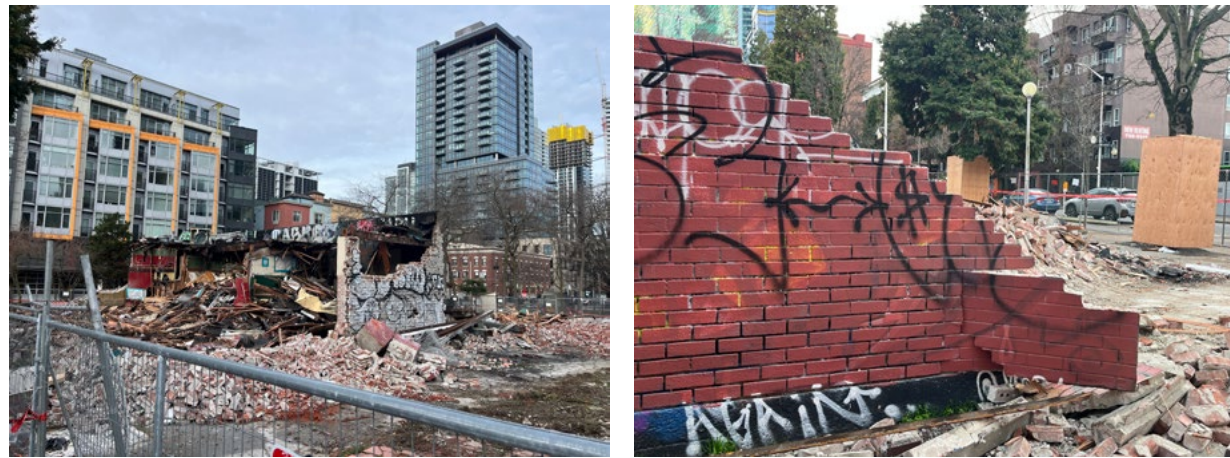
Figure 4.22 Demolition of building at 2234 2nd Ave, 'Mama's Mexican Kitchen.' Photos taken January 2, 2025.
