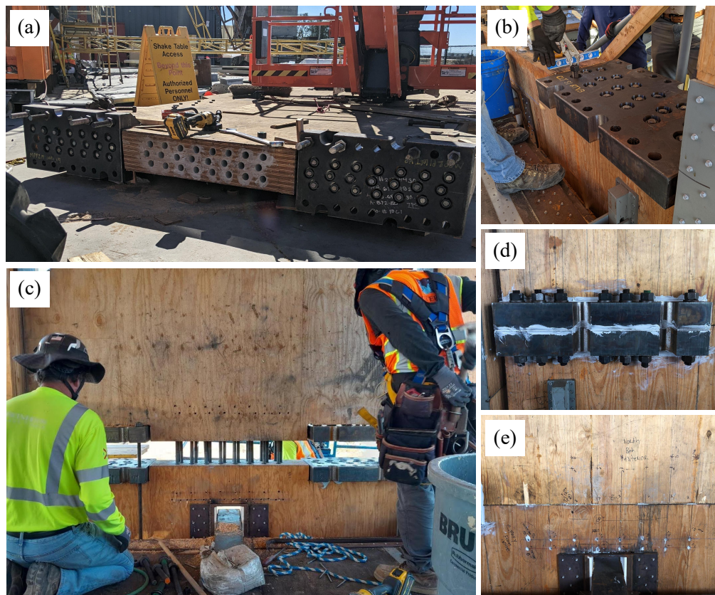
Figure 6.33: Shear wall splice installation procedure: (a) horizontal installation of splice plates on upper wall panels, (b) vertical installation of splice plates on lower wall panels and rod epoxying, (c) lowering of upper wall panel, (d) final tension rod and splice plates, and (e) final shear rods
