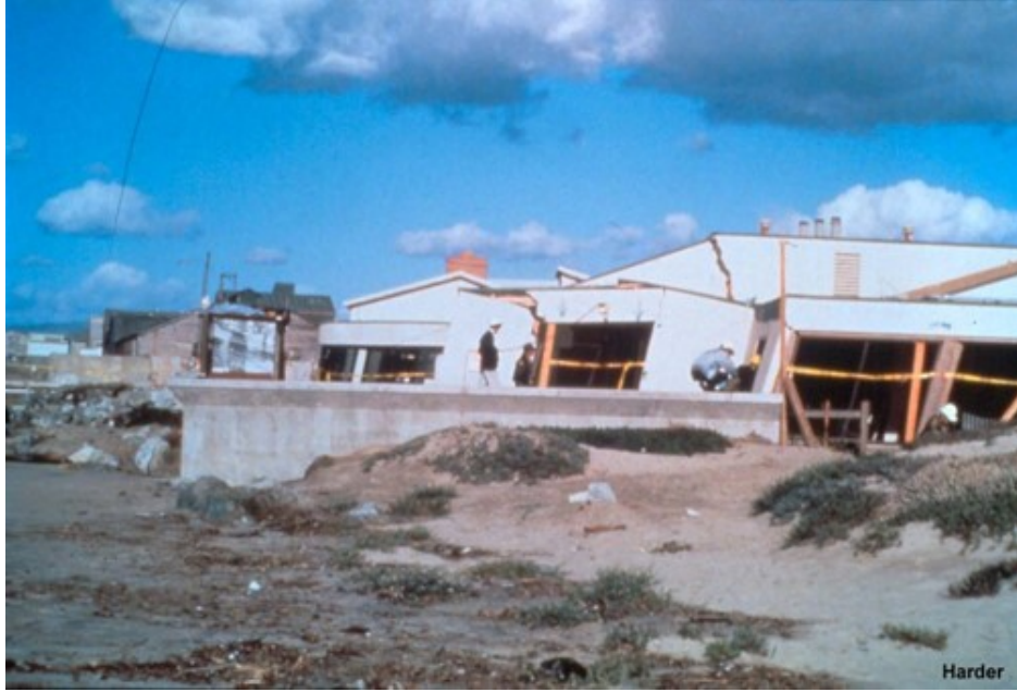
Figure 2.5: Damage to Marine Laboratory building in Moss Landing, CA, due to lateral spreading deformations of over 1 meter. (U.S. Geologic Survey)
