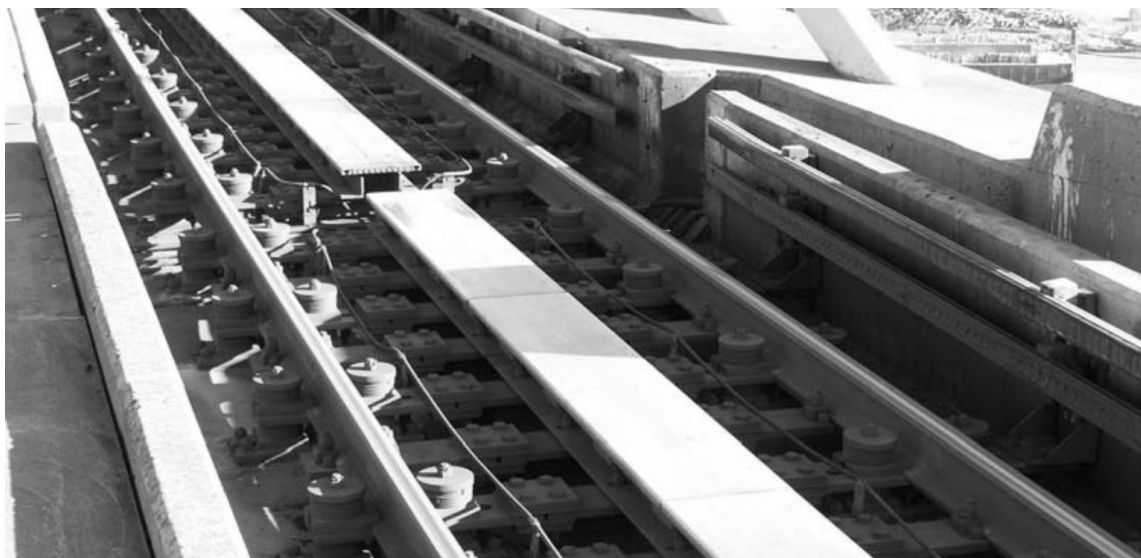
Figure 1-4: SkyBridge expansion joint picturing cylindrical elastomeric springs (Parsons Brinckerhoff, 2006).
