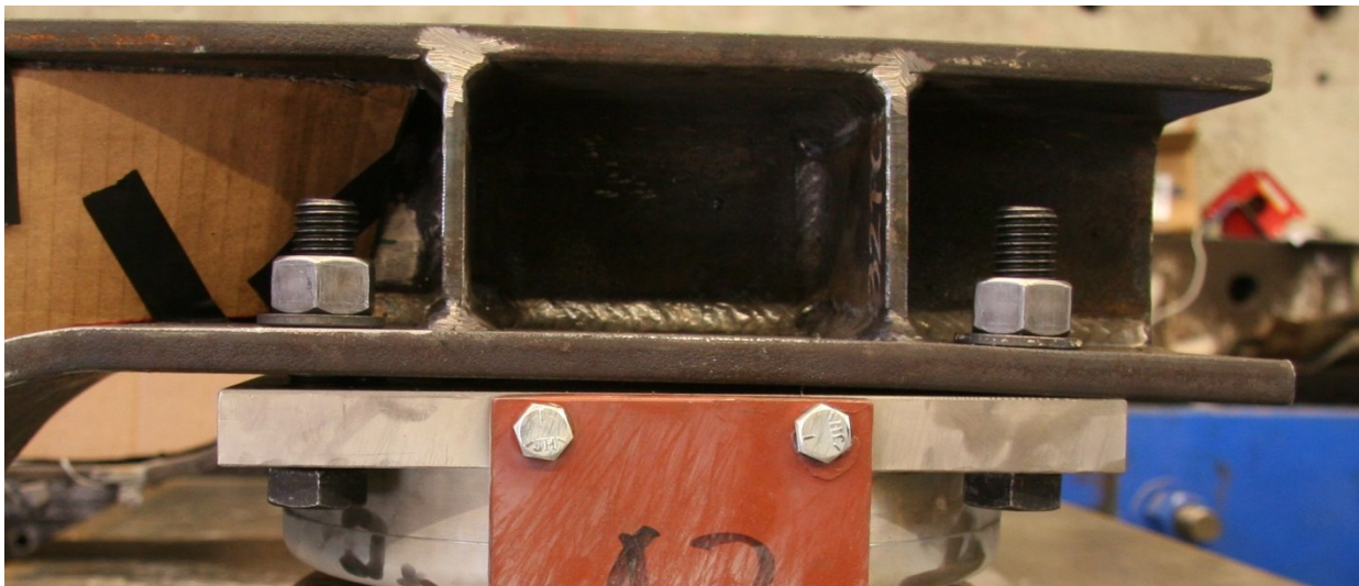
Figure 2-12: Bearer bar/bearing initial misfit ( NOTE: FPS bearing shipping plates are still attached ).
