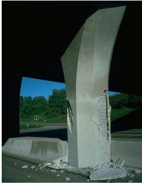
Figure 2.6: Unconfined concrete on the Ruffner Ave bridge spalled off during the 1994 Northridge earthquake [31].
