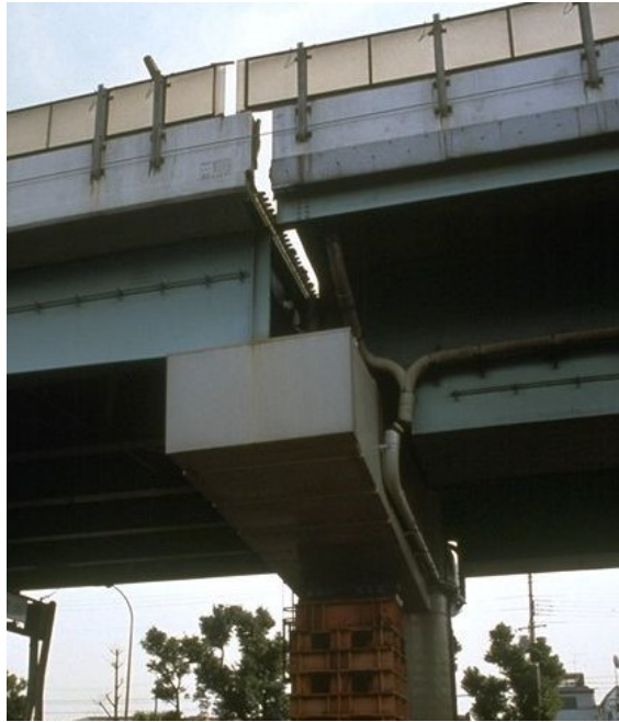
Figure 2.3: Differential movement between adjacent deck sections at an expansion joint led to a span discontinuity at pier 97 of the Hanshin Expressway in Japan after the 1995 Kobe Earthquake [55].
