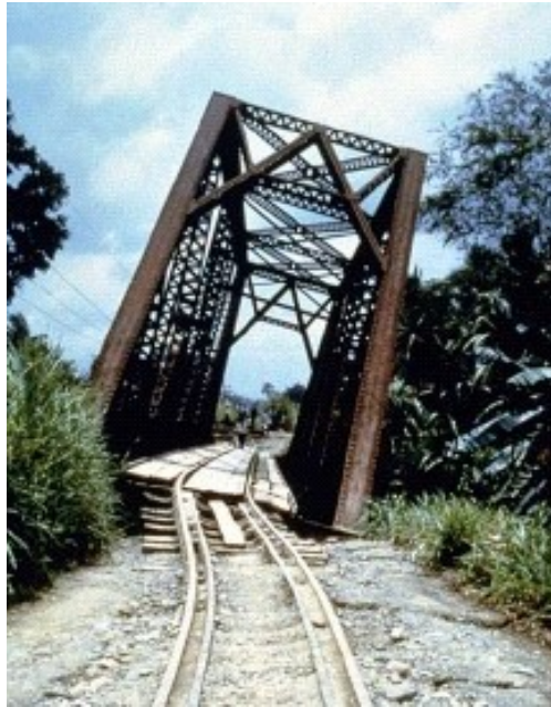
Figure 2.8: Lateral spreading around the foundations of a railroad bridge in Costa Rica during the 1991 Limon earthquake caused significant displacement of the structure [64].
