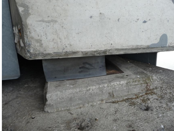
Figure 2.7: An unbolted elastomeric bearing supporting the Bridge Street bridge outside Christchurch experienced a sliding failure during the 2010 New Zealand earthquake [11].
