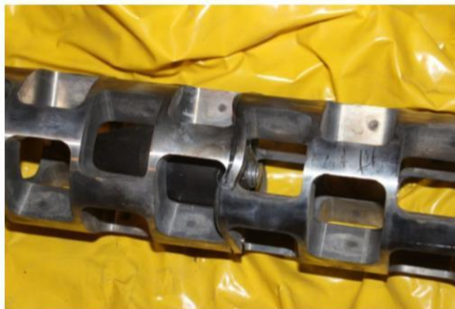
Figure 3. 5: Baffle local buckling
