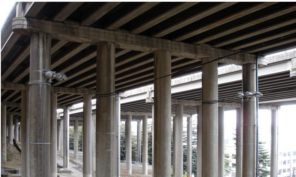
Figure 20: View from underneath the highway structure with spanning elements between columns supporting lighting and sprinkler features
