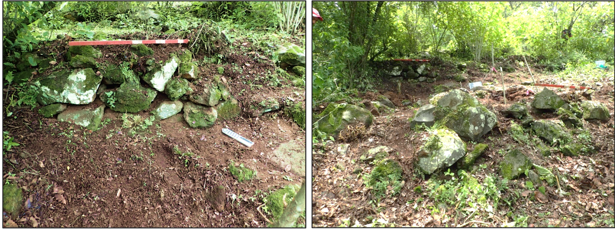
Figure 5.28. Left: photo of the stone wall. Only part of it is exposed due accumulation of sediment and collapse. Terrace is above stone wall. Right: the stone wall in background and the retention wall for the hill in foreground.
