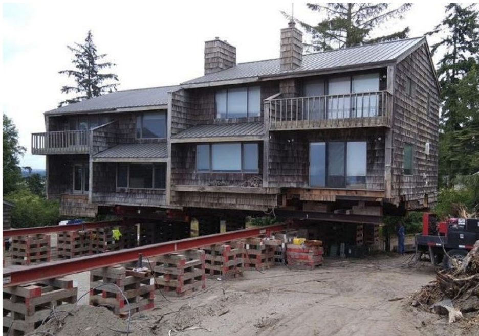
Figure 24. Photo of a building being moved back from the coastline performed by DB Davis Structural Moving & Raising Company.
