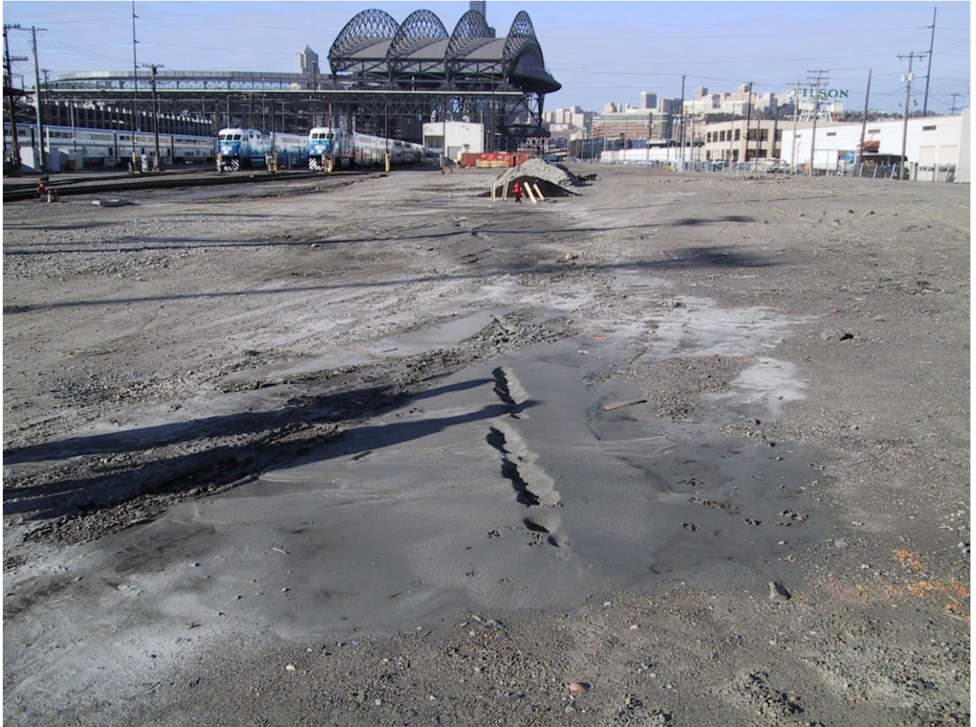
Figure 4- Photo of sand boils (location 7) south of T-Mobile Park in the railyard between S Massachusetts St and S Holgate St. Photo provided by Kathy Troost.
