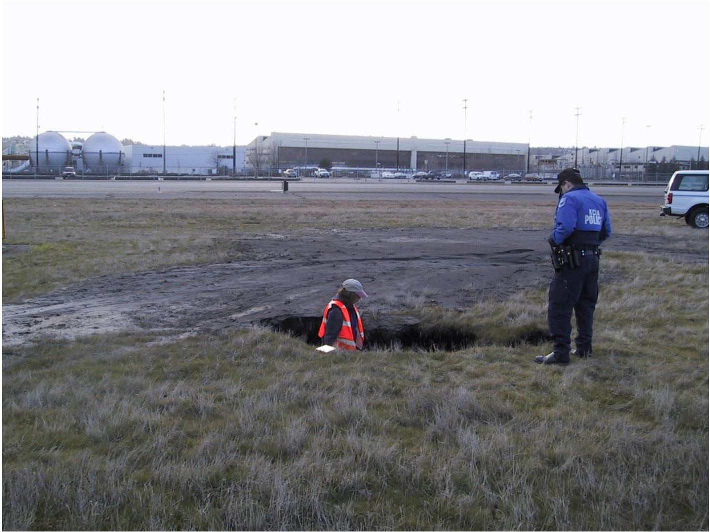
Figure 3- Photo of sinkhole and sand boils at Boeing Field following the Nisqually earthquake. Half of Kathy Troost for scale. Photo provided by Kathy Troost.
