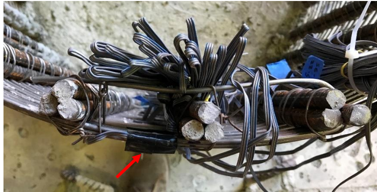
Figure 5.18: Overhead view of uppermost wire strain gauge on the south end of the shaft reinforcement cage (indicated by red arrow; photo was taken mid-installation)
