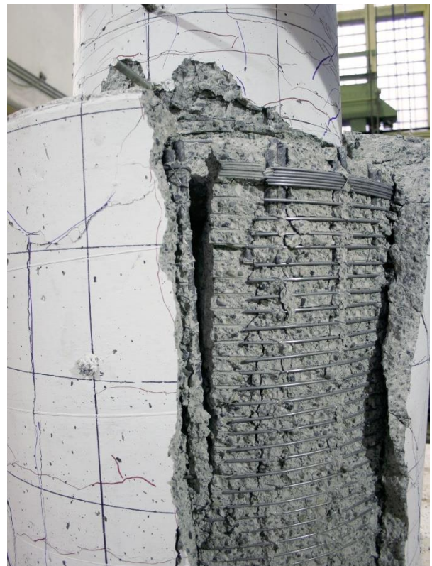
(b) Line of spiral fracture on southeast side
