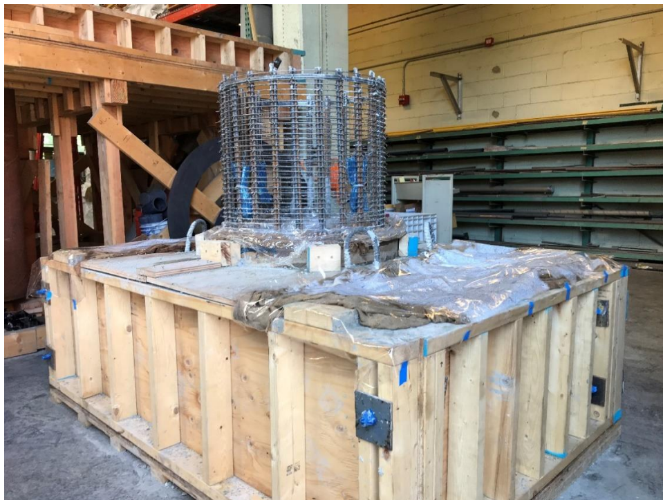
Figure B.3: End of first concrete placement (base and shaft starter stub)
