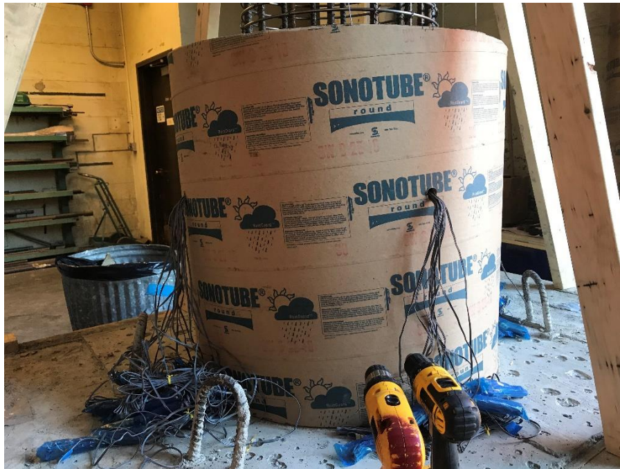
Figure B.4: Sonotube formwork for the shaft, with strain gauge leads routed out
