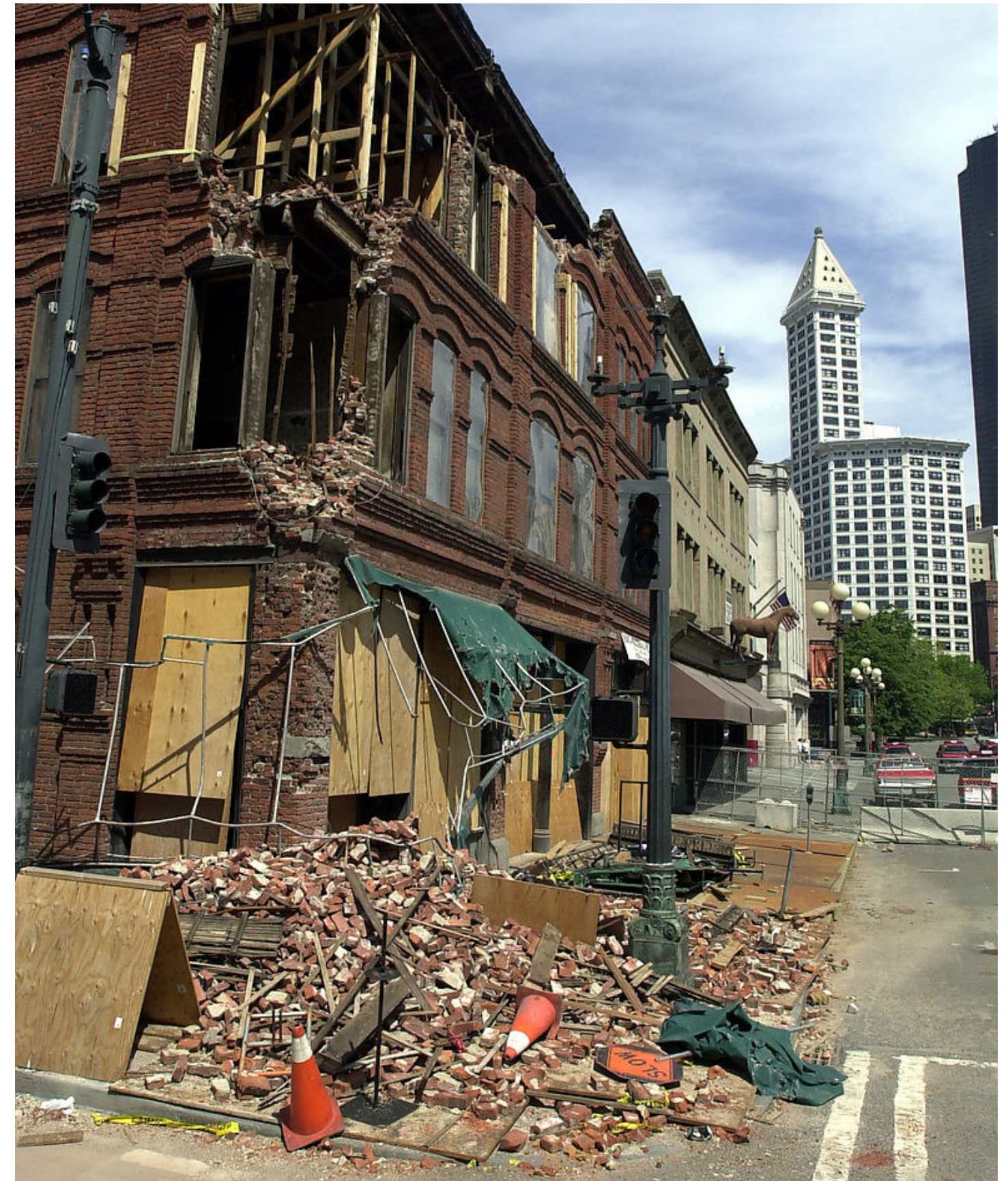
Figure 2.10 Damage to the Cadillac Hotel in Pioneer Square after the 2001 Nisqually Earthquake (Photo courtesy of Erik Stuhaug from the Seattle Municipal Archives)
