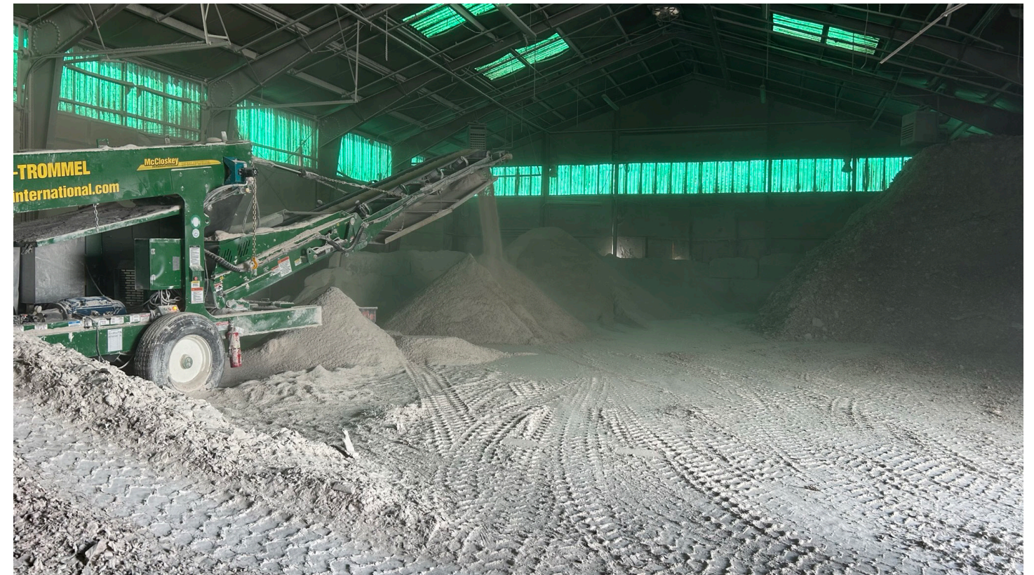
Figure 8.14 Drywall being ground down into an aggregate size at Gypsum to Gypsum’s recycling center in the South Park neighborhood of Seattle (Photo by author)
