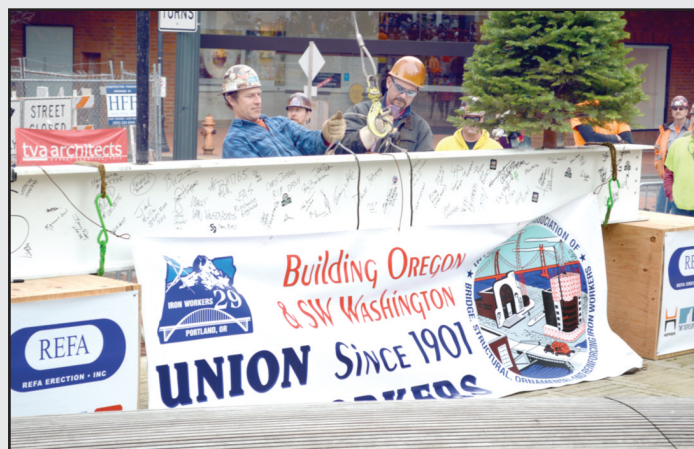
Local 29 ironworkers James Marble and Doug Green attach the final steel beam to a cable from a tower crane operated by Anson Barrow of Operating Engineers Local 701.
