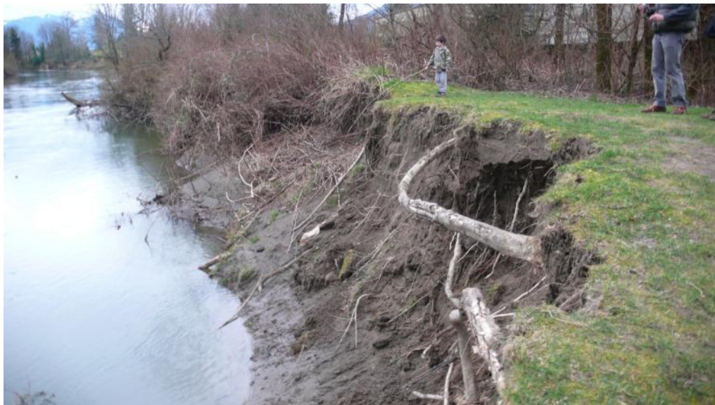
Figure34. Current erosion in Snoqualmie River bank at Sandy Cove Park . Shot by Pin-hao, Huang. (March2014).
