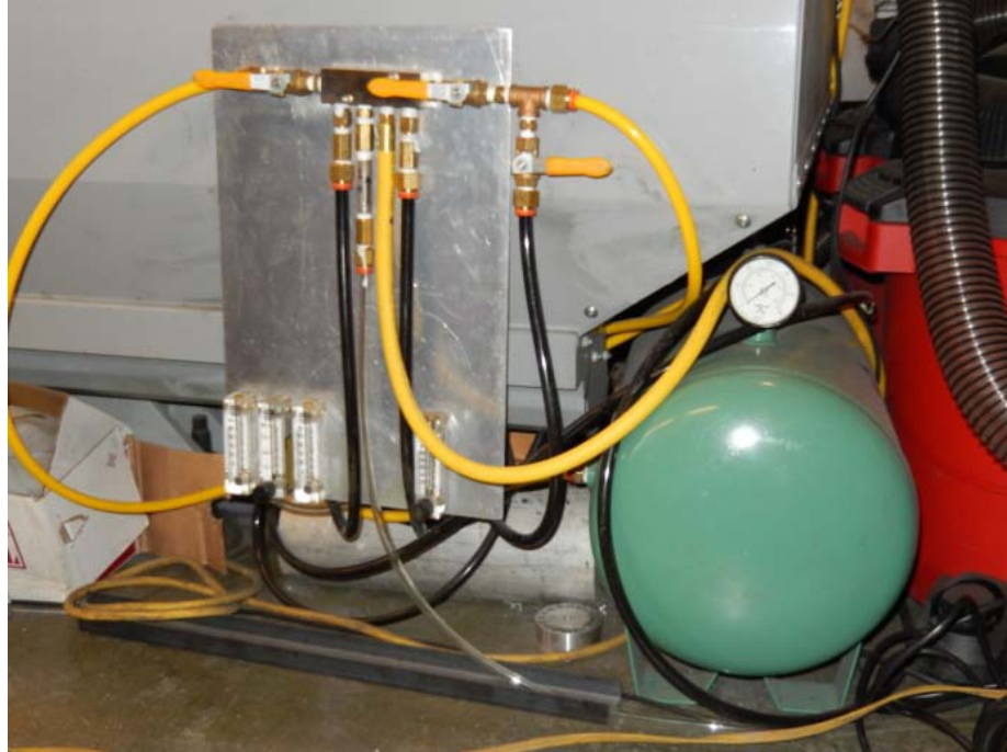
Figure 3-19: Vacuum pump and Manifold
