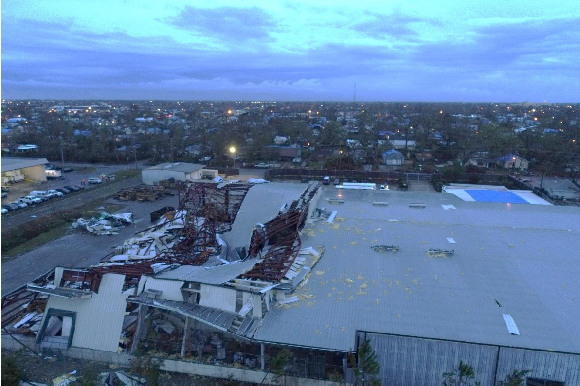
Figure 3.35. Overview of the damages to Miller Distribution Center.
