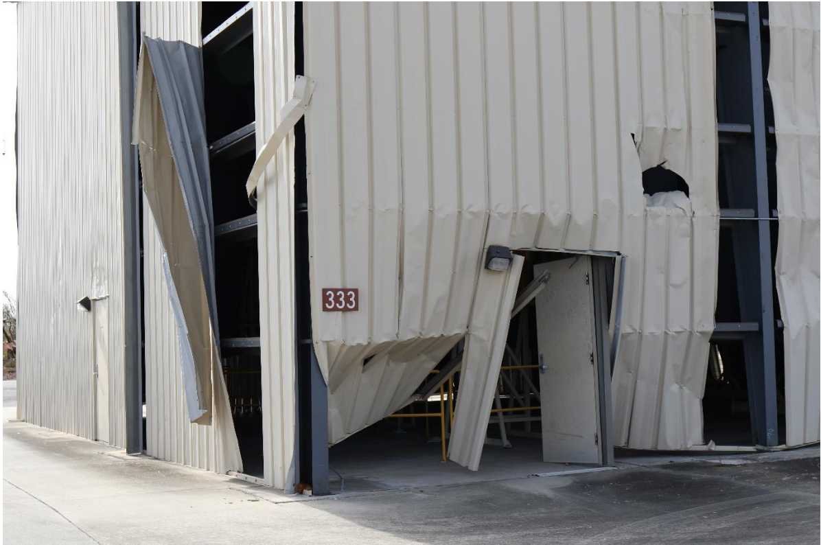
Figure 3.27. Paneling damages to Building 333.
