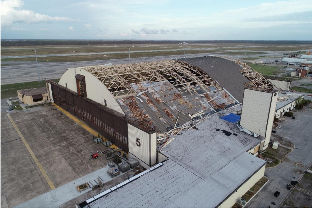
Figure 3.22. Overview of roof damage on the south facing side of Hangar 5.
