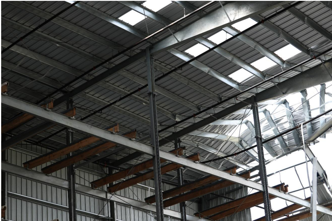
Figure 3.12. A view of the buckled purlins of Watson Landings Marina.
