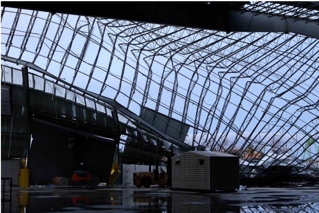
Figure 3.8. A photograph showing the buckled roof trusses in Westrock East Terminal.
