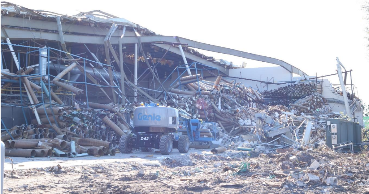
Figure 3.33. View of the collapsed beam in Parthenon.
