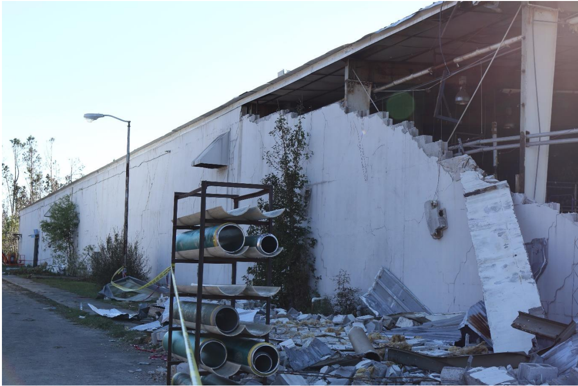
Figure 3.34. View of the damaged wall in Parthenon.
