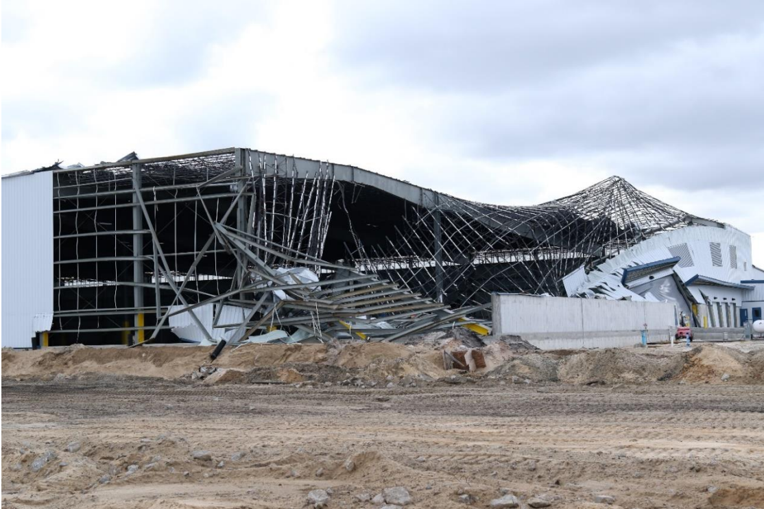
Figure 3.7. A view of the damaged face of Westrock East Terminal.
