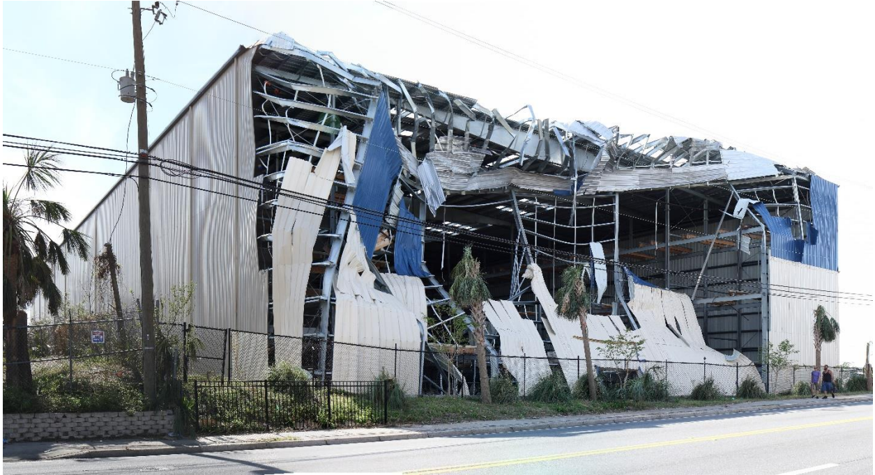
Figure 3.11. A view of the damaged face of Watson Landings Marina.
