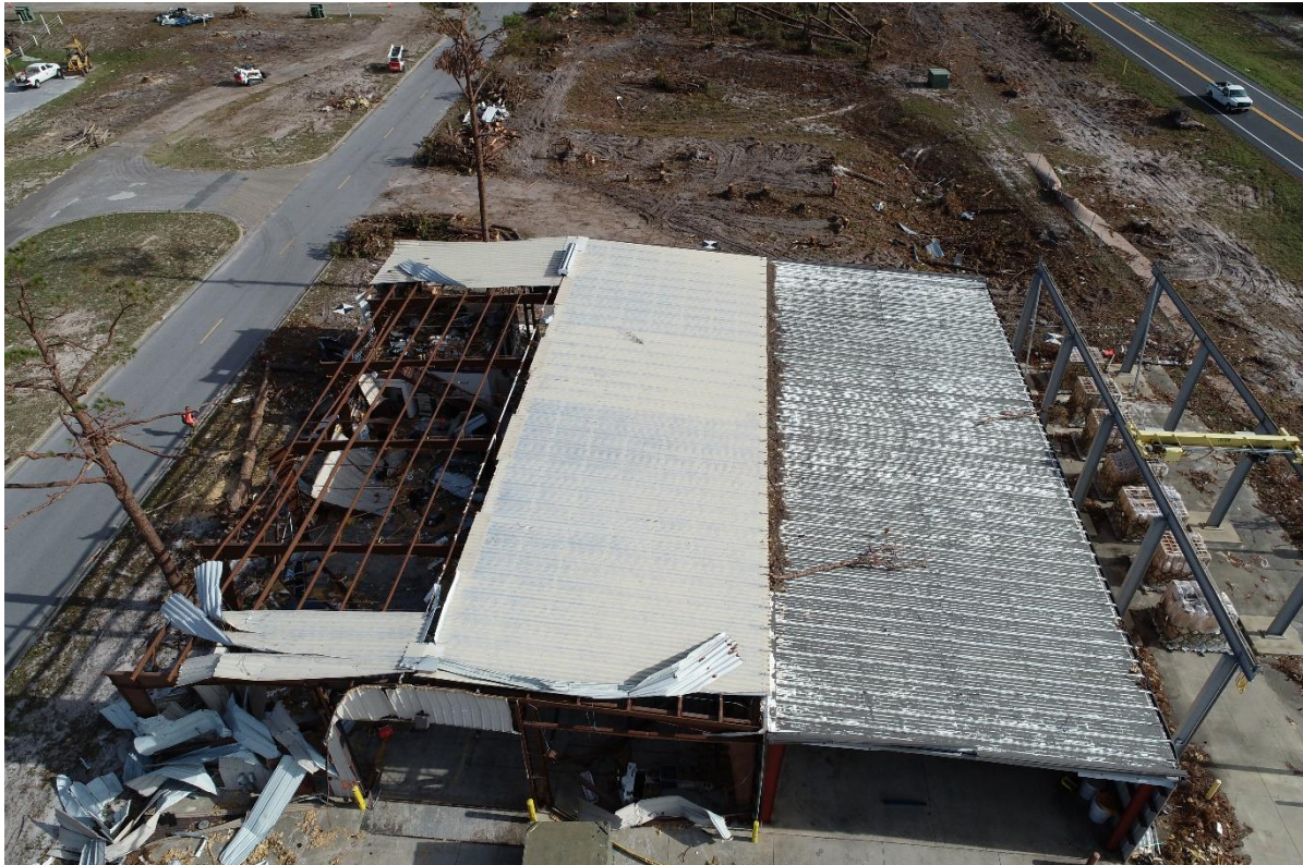
Figure 3.30. The roof damage to Building 375.
