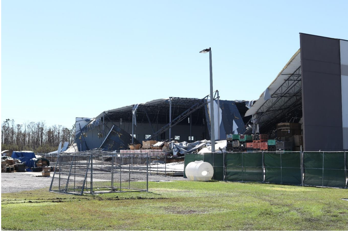
Figure 3.15. The damaged face of the IDC.
