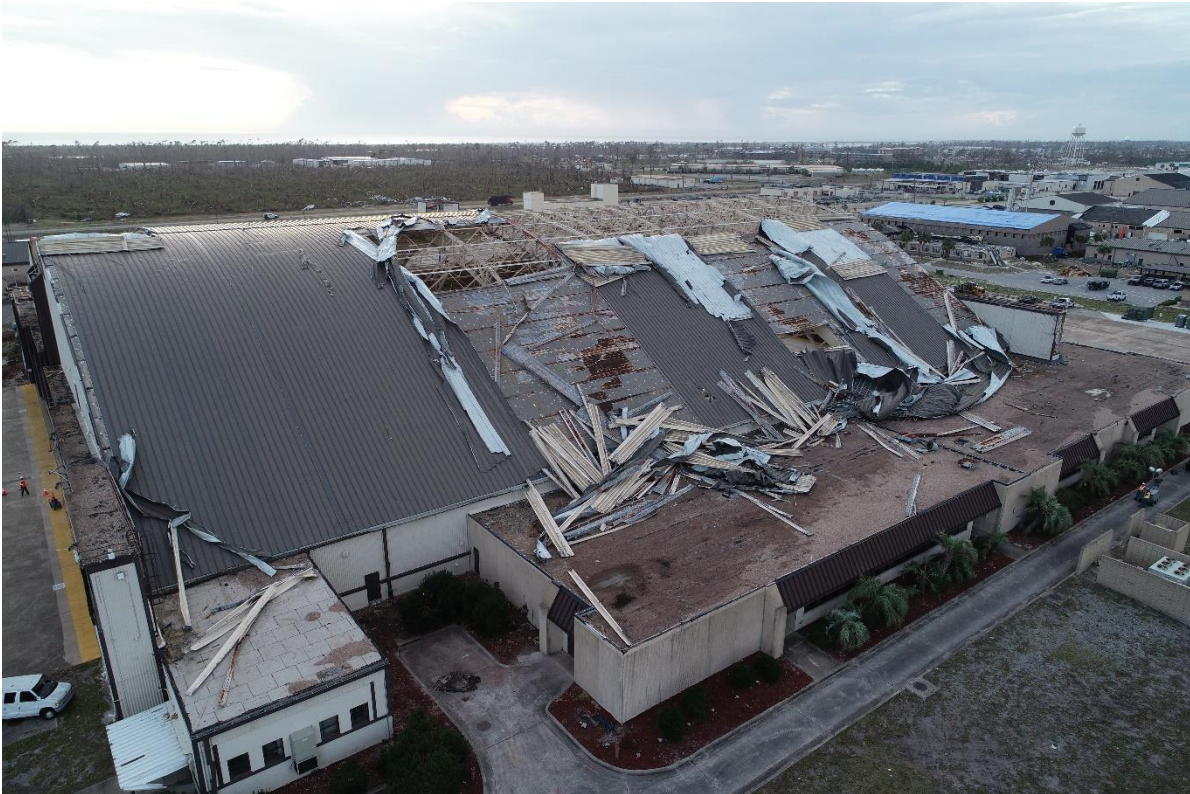
Figure 3.23. Overview of roof damage on the north facing side of Hangar 5.
