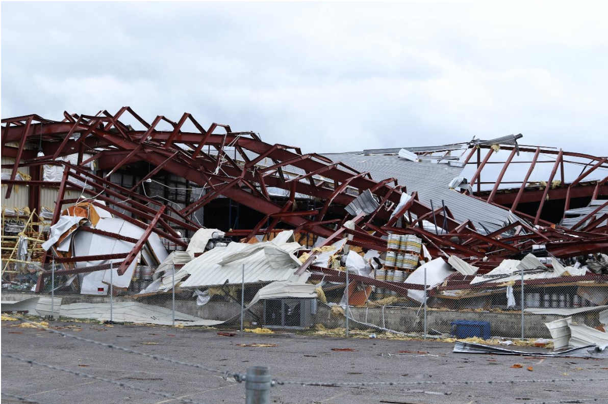
Figure 3.36. Another view of the damages to Miller Distribution Center.
