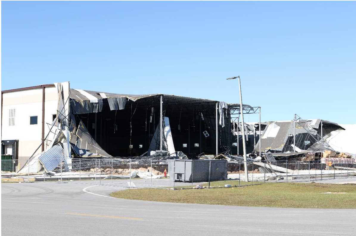
Figure 3.16. The damaged face of the IDC.
