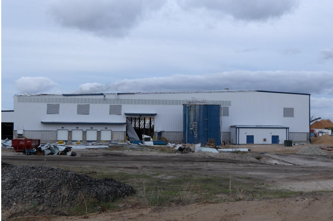
Figure 3.5. A view of the intact face of Westrock East Terminal demonstrating the off-center roof pitch.
