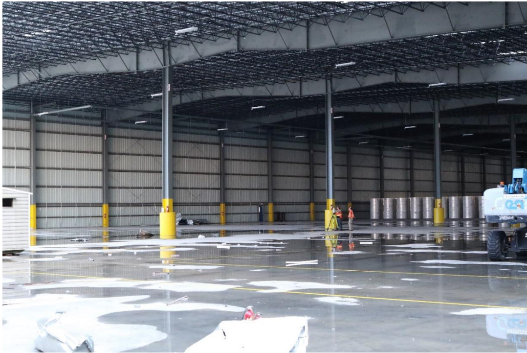
Figure 3.6. A view from inside Westrock East Terminal showing the framing and columns.
