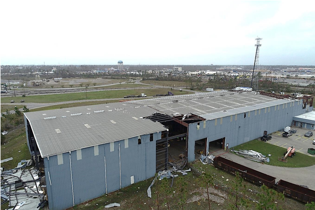
Figure 3.19. Other damage to Cargill Distribution Center.
