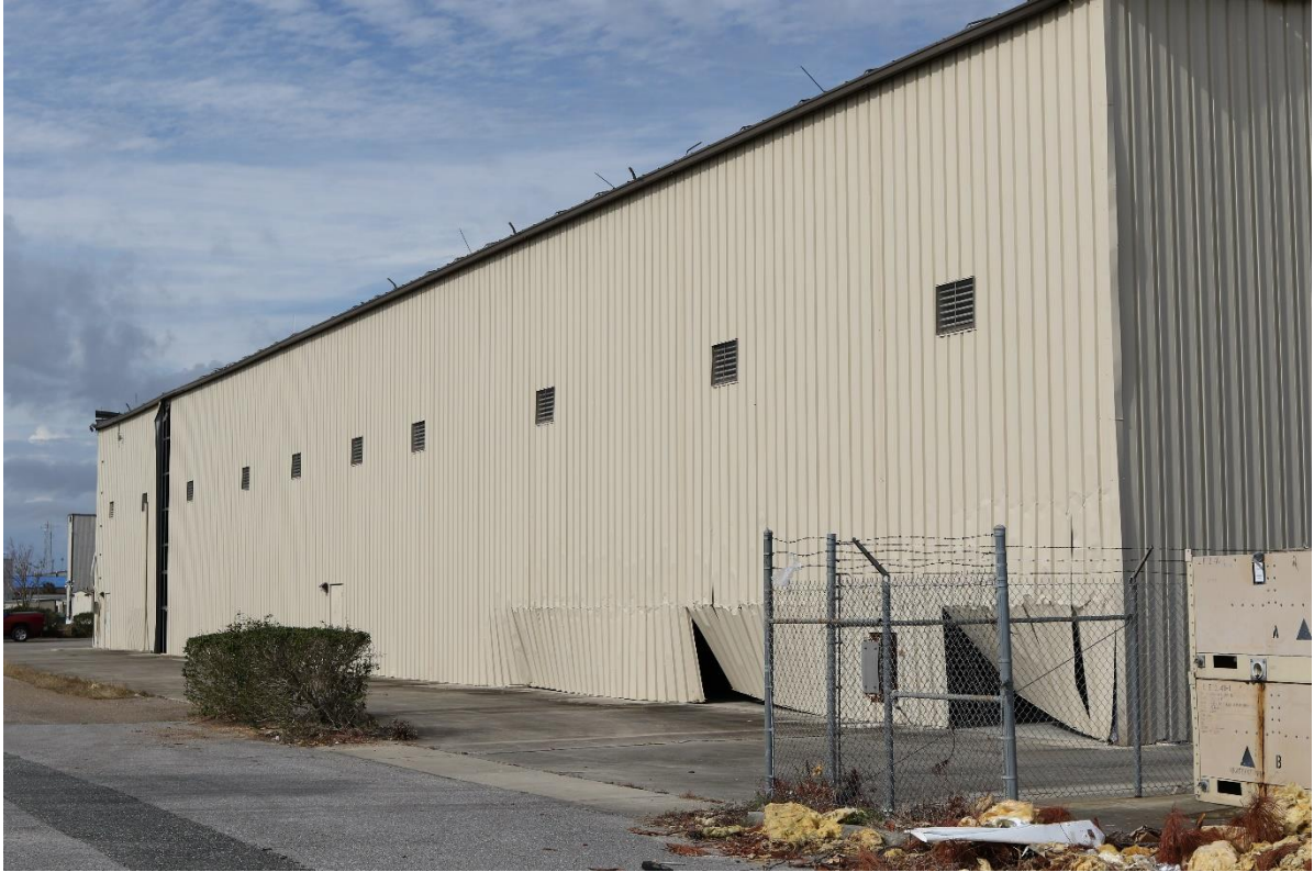
Figure 3.28. More paneling damages to Building 333.
