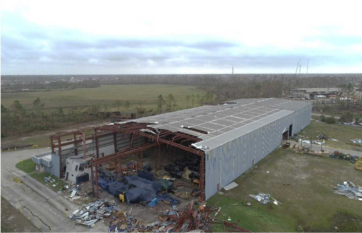
Figure 3.18. The collapsed side of Cargill Distribution Center.
