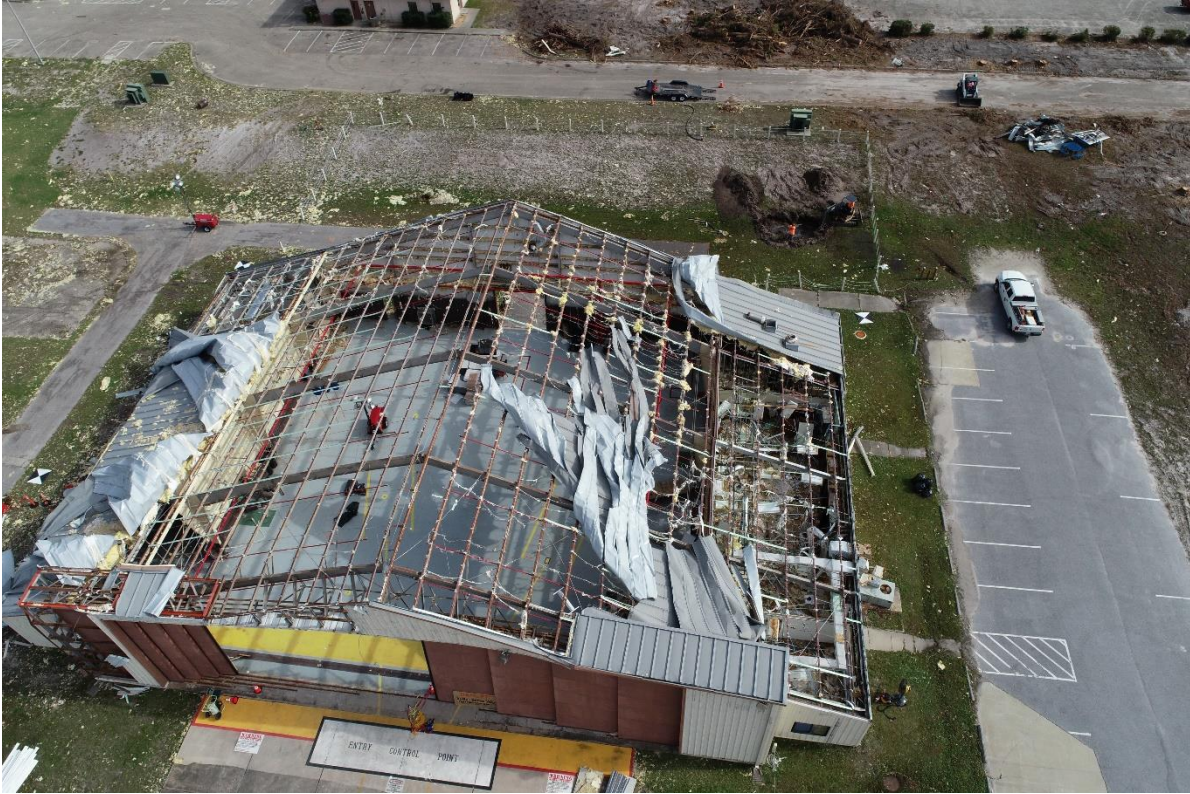
Figure 3.25. The roof damage to Building 316.
