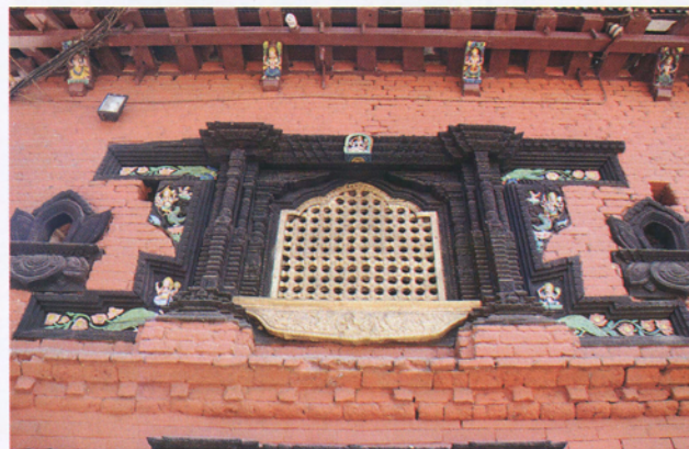
Figure 10: Harasiddhi temple golden temple window on north side of temple. Recently painted over with gold paint. (photo Arun Maharjan)
