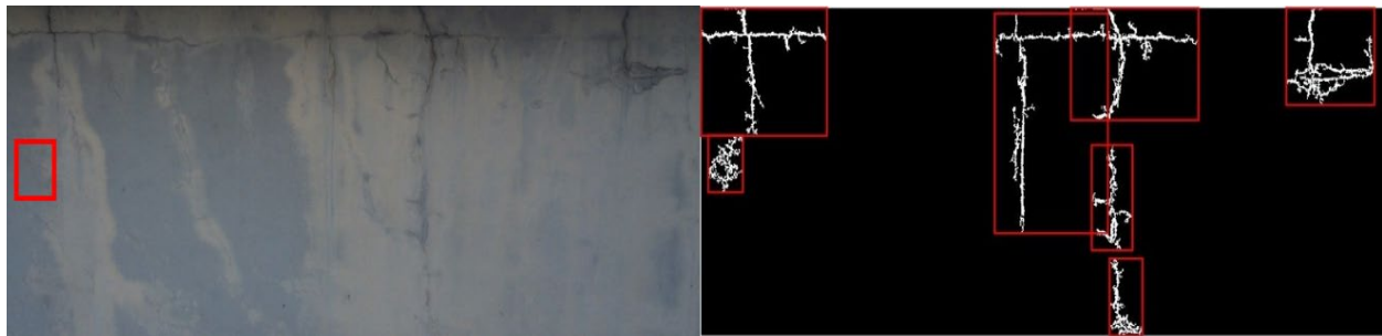
Figure 5.7 Crack detection results: (a) Original UAS image; (b) Detected and labeled cracks on the UAS image
