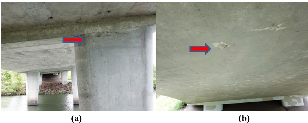
Figure 5.2 (a) Sacking is falling off of a column; (b) Spalling at the bottom of the girder box
