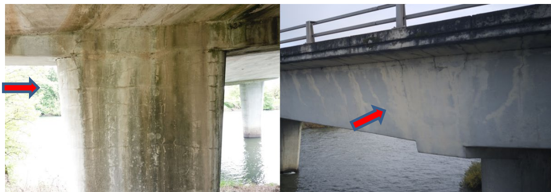
Figure 5.1 (a) Hairline shrinkage cracks on a column; (b) Hairline flexure cracks with efflorescence on the sides of boxes
