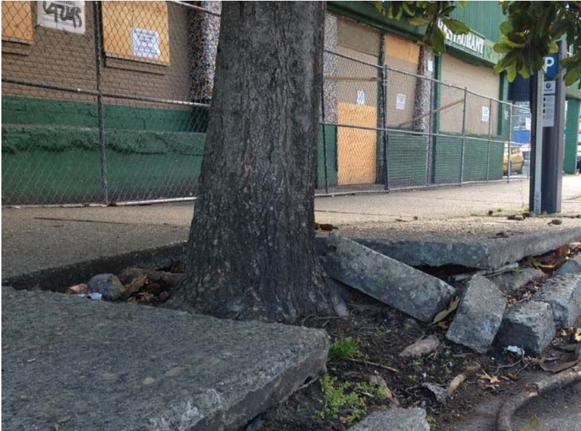
Photo 4.1: Sidewalk upheaval is common in Seattle.
