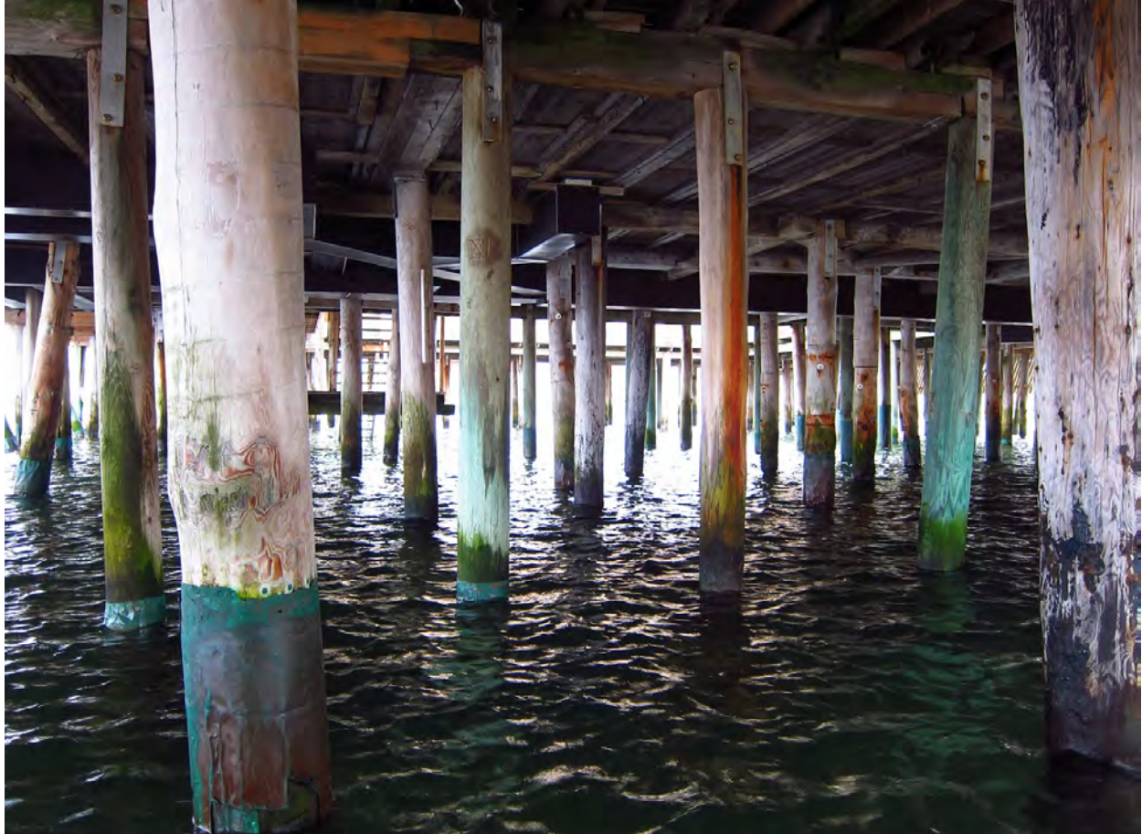
A tangle of piers support Varbergs Kallbadhus, similar to those at Ribersborg. Image Source: Jesce Walz
