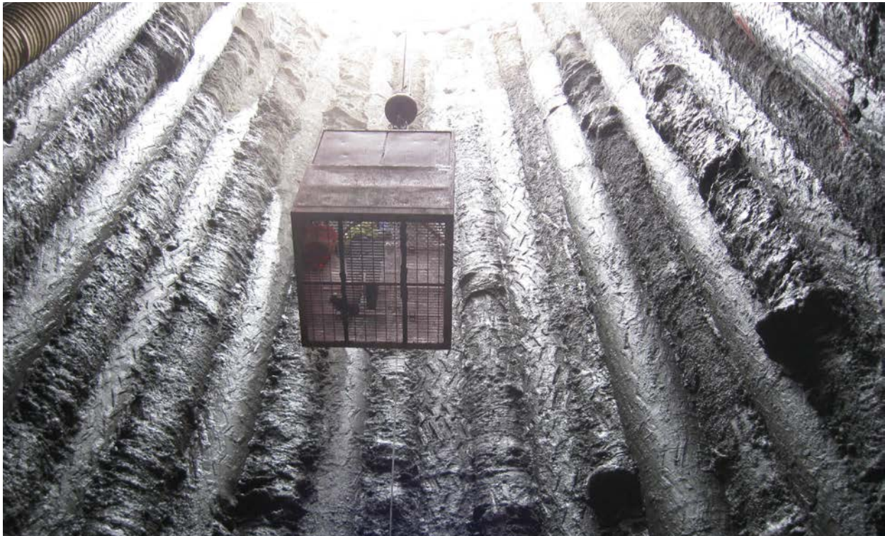
Fig. 2.12: Workers being lowered into the access way for Ballard Siphon, which directs combined stormwater and sewage from the north side of the Ship Canal to the West Point Treatment Plant (via Seattle Public Utilities)
