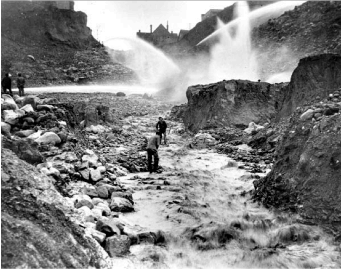
Figure 9. Regrading at Bell Street and Fourth Avenue. Hydraulic nozzles called ‘Giants’ were modified to allow for vertical and horizontal movement, and with a diameter of 2.5-3.5 inches created water pressures of 75-100 pounds per square inch. The Giants could consume up to 12 million gallons of water a day, a third of the Cedar River supply (Karvonen 2010). Image Source: University of Washington Libraries Special Collections, Lee 20022 (in Karvonen 2010).
