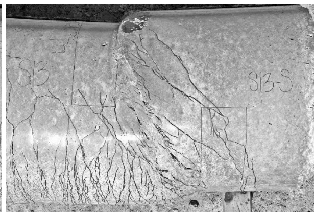
f) Specimen 13 south span concrete cracking
