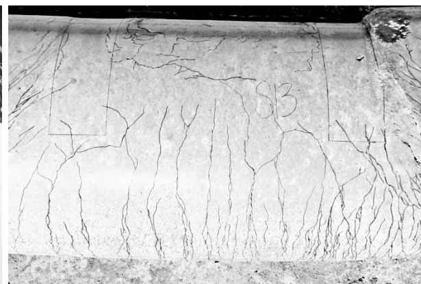
d) Specimen 13 mid-span concrete cracking
