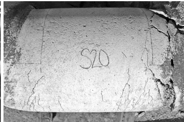
d) Specimen 20 mid-span concrete cracking
