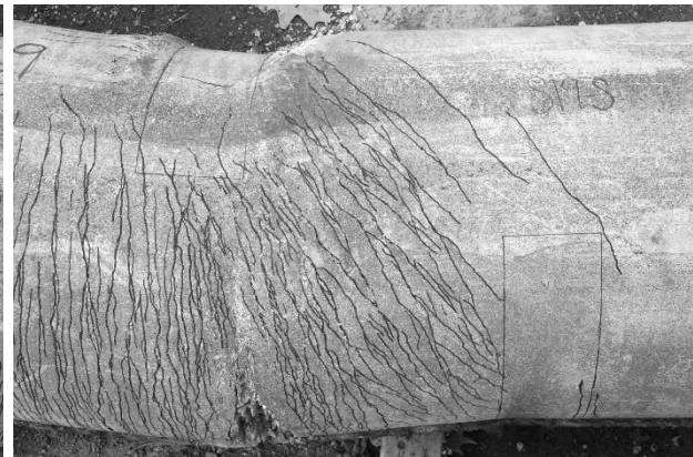
f) Specimen 19 south span concrete cracking
