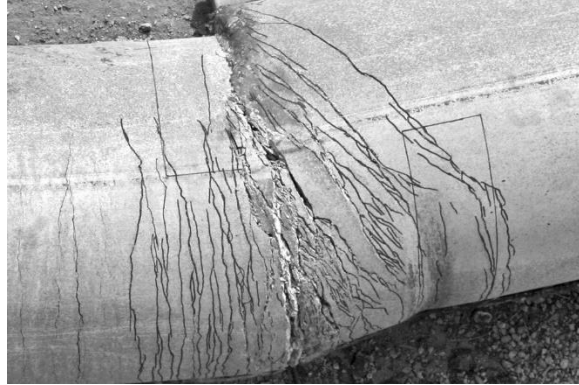
Figure 5.10: Extensive shear cracking
