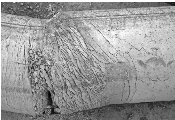
f) Specimen 12 south span concrete cracking
