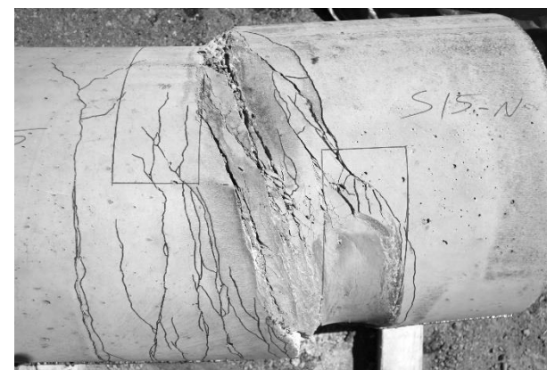
f) Specimen 15 north span concrete cracking
