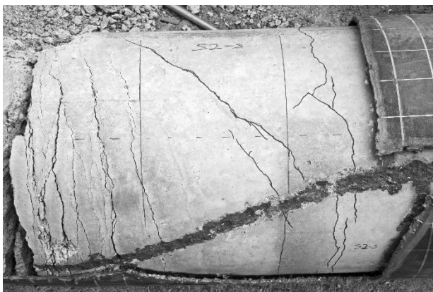
f) Specimen 2 south span concrete cracking
