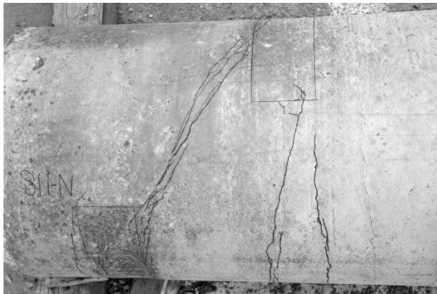
e) Specimen 11 north span concrete cracking
