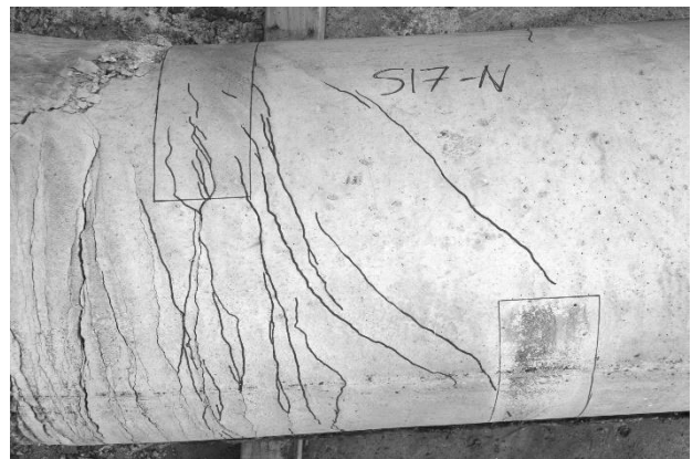
f) Specimen 17 north span concrete cracking
