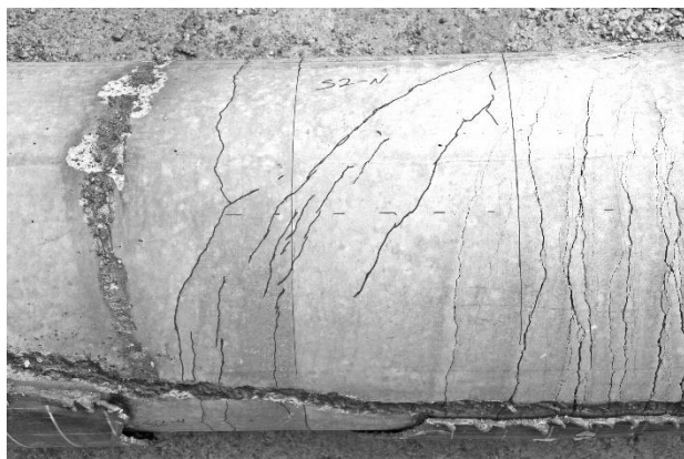
e) Specimen 2 north span concrete cracking
