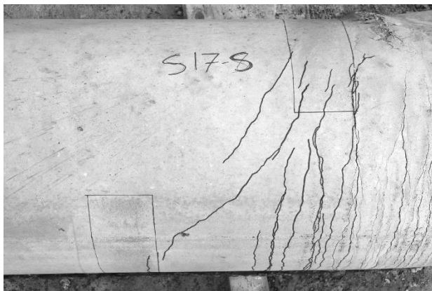
e) Specimen 17 south span concrete cracking
