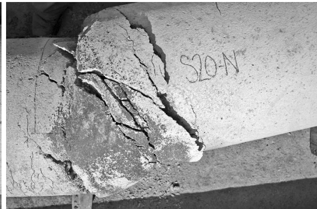
f) Specimen 20 north span concrete cracking
