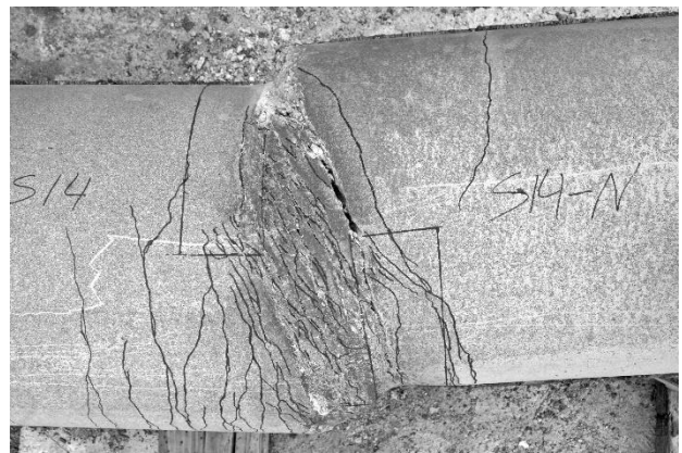
f) Specimen 14 north span concrete cracking
