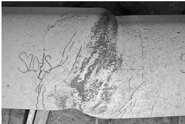
e) Specimen 20 south span concrete cracking
