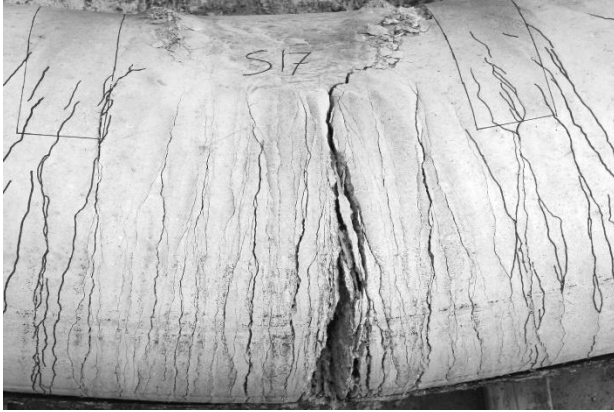
Figure 5.2: Dense flexural cracking
