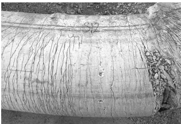
d) Specimen 12 mid-span concrete cracking
