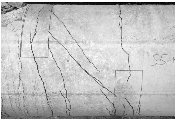
f) Specimen 5 north span concrete cracking
