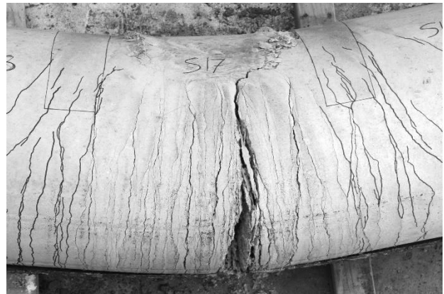
d) Specimen 17 mid-span concrete cracking
