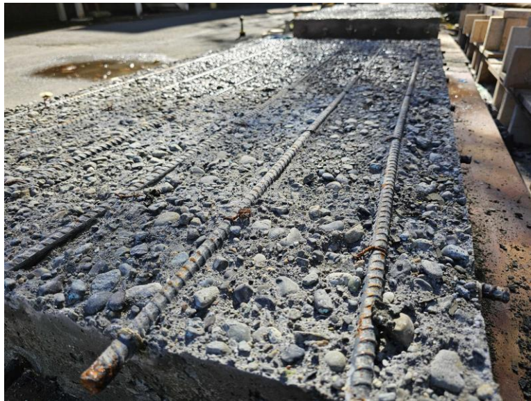
Figure A.15: Picture of Exposed Aggregate Etching on “Significantly Deteriorated” Deck
