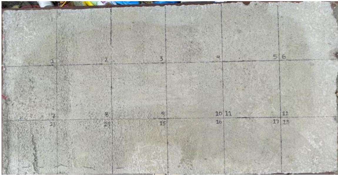
Figure A8: First assessment cracks of Deck 5 – Exposed Rebar, CSAP
