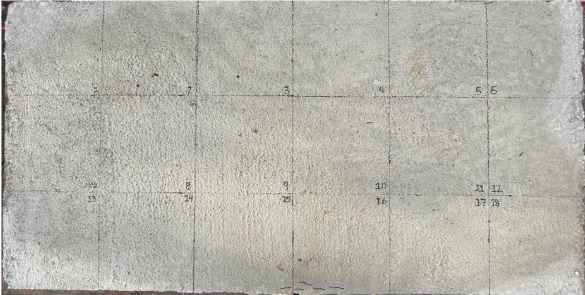
Figure A6: First assessment cracks of Deck 3 – Exposed Aggregate, CSAP
