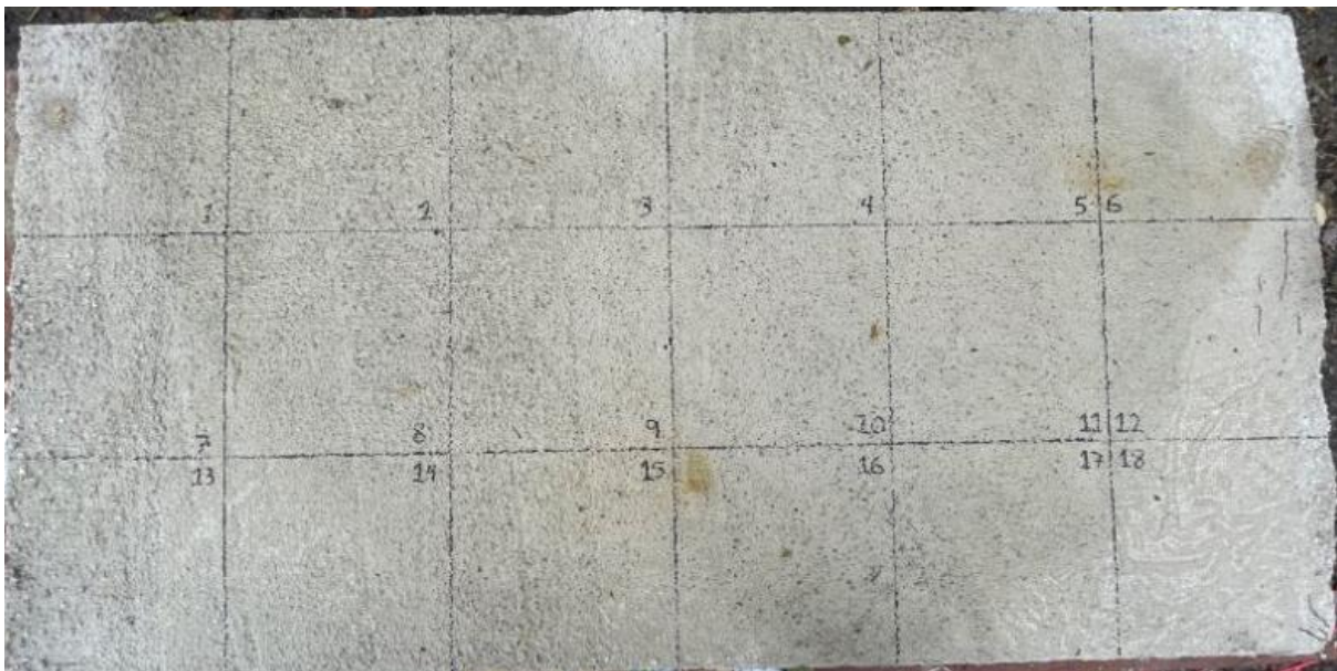
Figure A9: First assessment cracks of Deck 6 – Exposed Aggregate, CSAP
