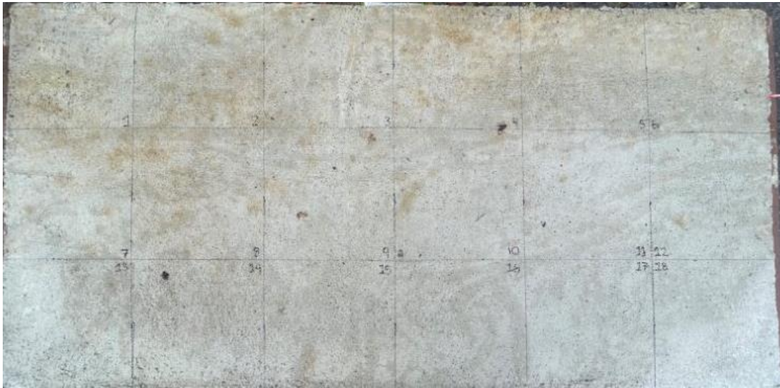
Figure A4: First assessment cracks of Deck 1 – Sandblasted, CSAP
