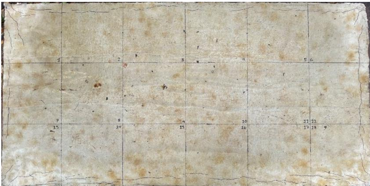
Figure A5: First assessment cracks of Deck 2 – Sandblasted, LLP
