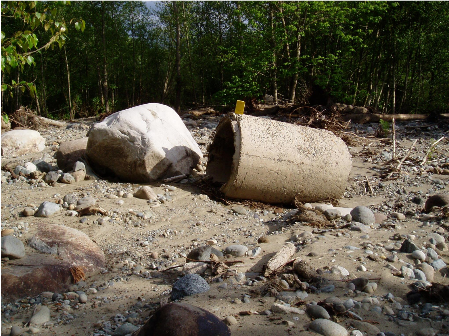
Figure 4a: Image of a concrete culvert that was blown out and transported downstream by the failure of a beaver dam upstream of the Snoqualmie Valley Trail in King County in 2005. Notebook is 7 inches tall. (Source: John Bethel. Accessed: 2017).
