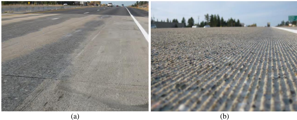
Figure 1-3. (a) Wheel path PPC inlay, (b) PPC overlay with diamond grinding (Anderson et al. 2013)
