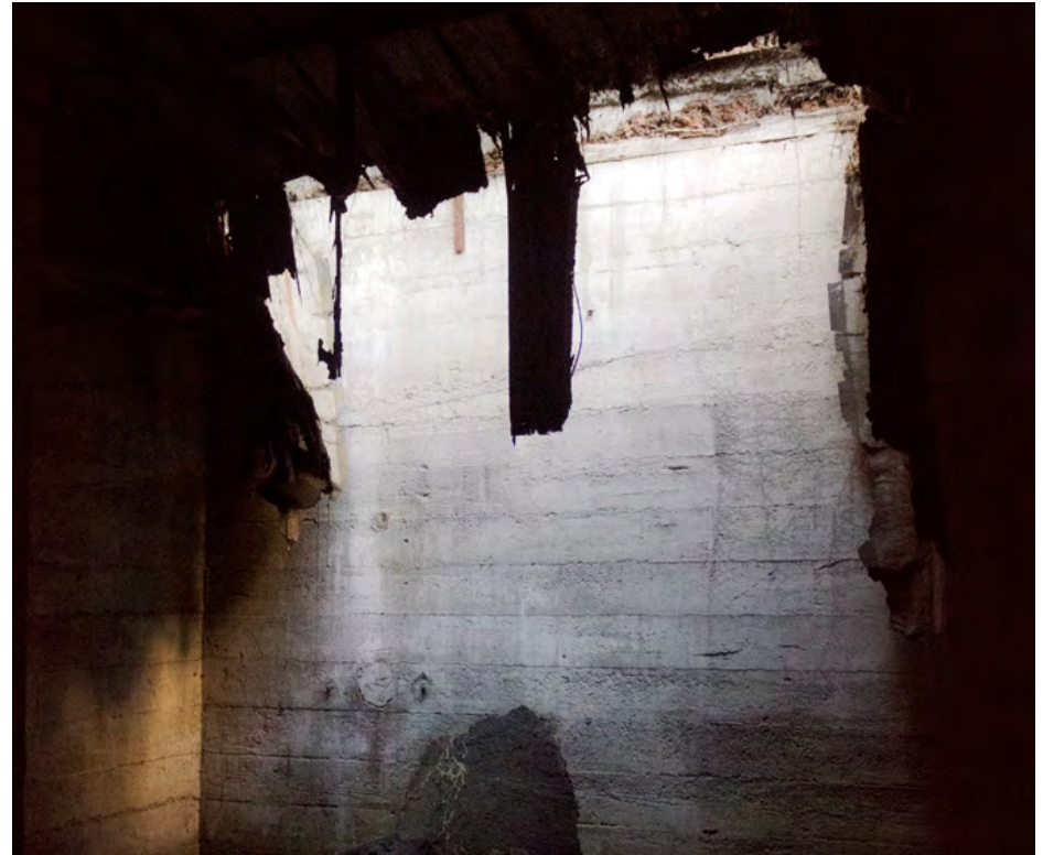
Figure 24: The sublime result of a roof collapse in Mill 1&2
