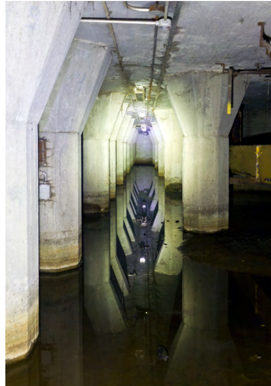
Figure 16: Basement flooding *For additional site photos see a Appendix A
