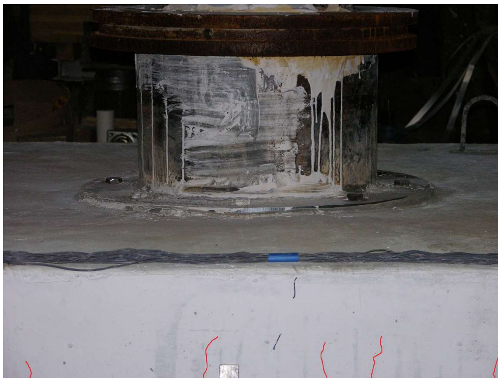
Figure 6.3. Cracking on North Face of Slab – 500 kips (PTB_4.5_1_0_P)
