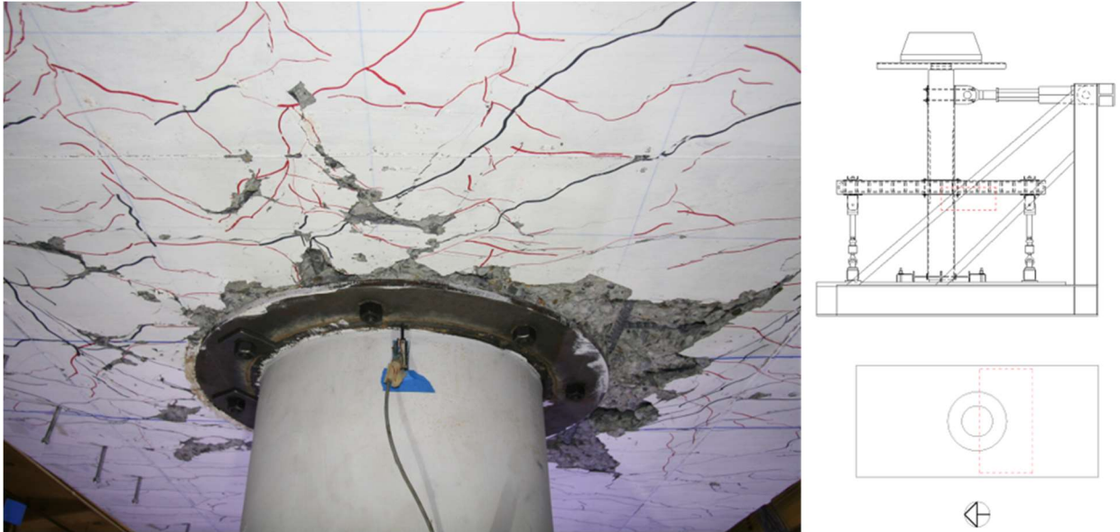
Figure 4.29. Damage on South Side of Bottom Face – 6.35% Drift (PTB_4.5_1_0_6)
