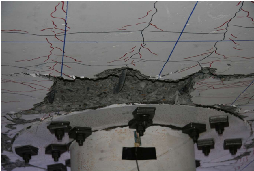
Figure 4.48. Bar Buckling on South Side of Bottom Face– 5.61% Drift (PTB_9_2_0_6)
