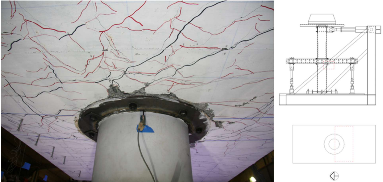
Figure 4.21. Crushing on South Side of Bottom Face – 4.91% Drift (PTB_4.5_1_0_6)
