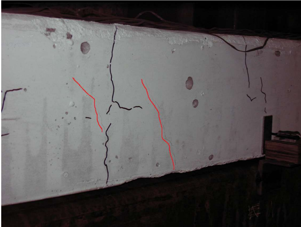
Figure 6.18. Cracking on North Face of Slab – 470 kips (PTB_9_2_0_P)
