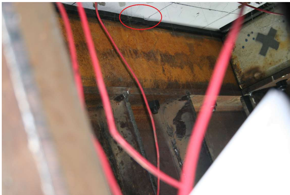
Figure 6.21. Cracking on Bottom Face of Slab near North Support – 670 kips (PTB_9_2_0_P)
