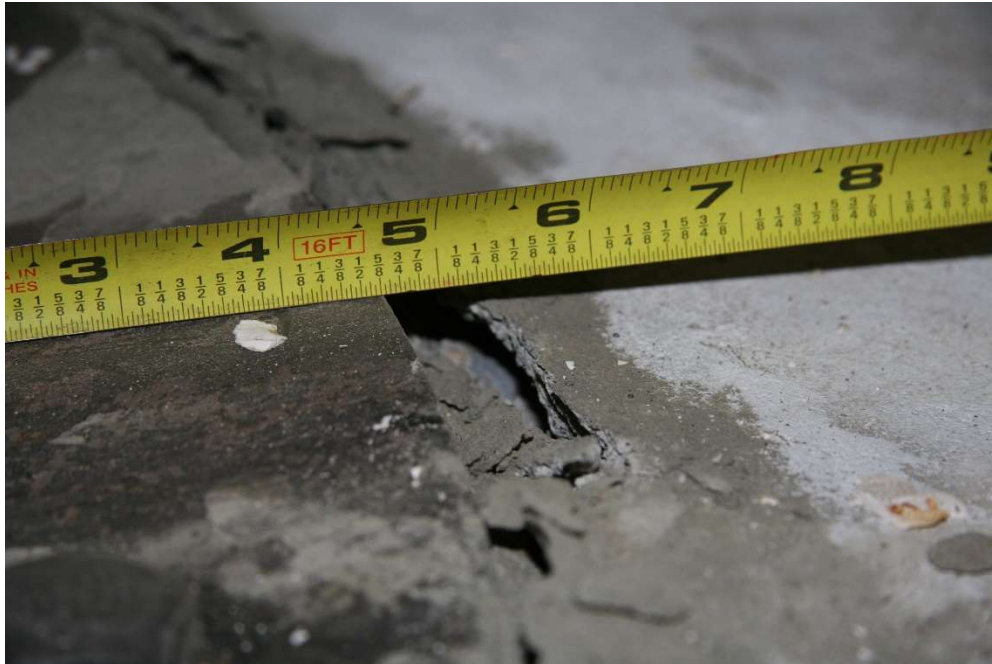
Figure 6.36. Southwest Side of Ring Flange – After Test (PTB_9_2_0_P)
