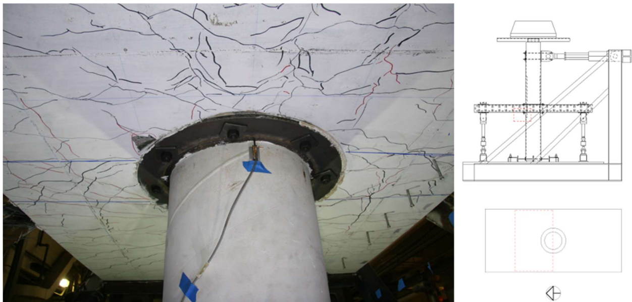
Figure 4.16. Spalling on North Side of Bottom Face – 3.48% Drift (PTB_4.5_1_0_6)
