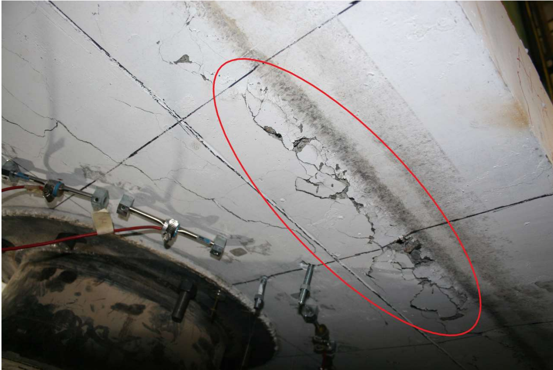
Figure 6.14. Spalling at North Support – Post Test (PTB_4.5_1_0_P)
