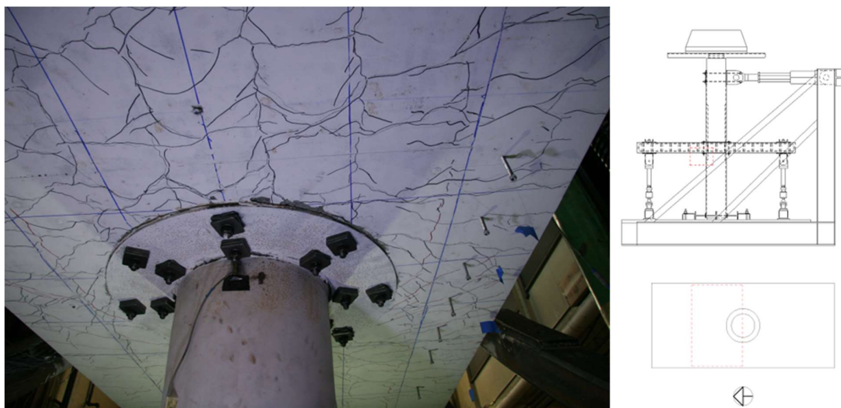
Figure 4.39. Spalling on North Side of Bottom Face– 3.54% Drift (PTB_9_2_0_6)
