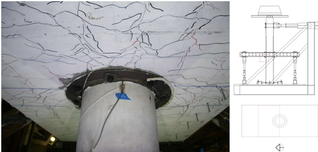
Figure 4.3. Example of Spalling
