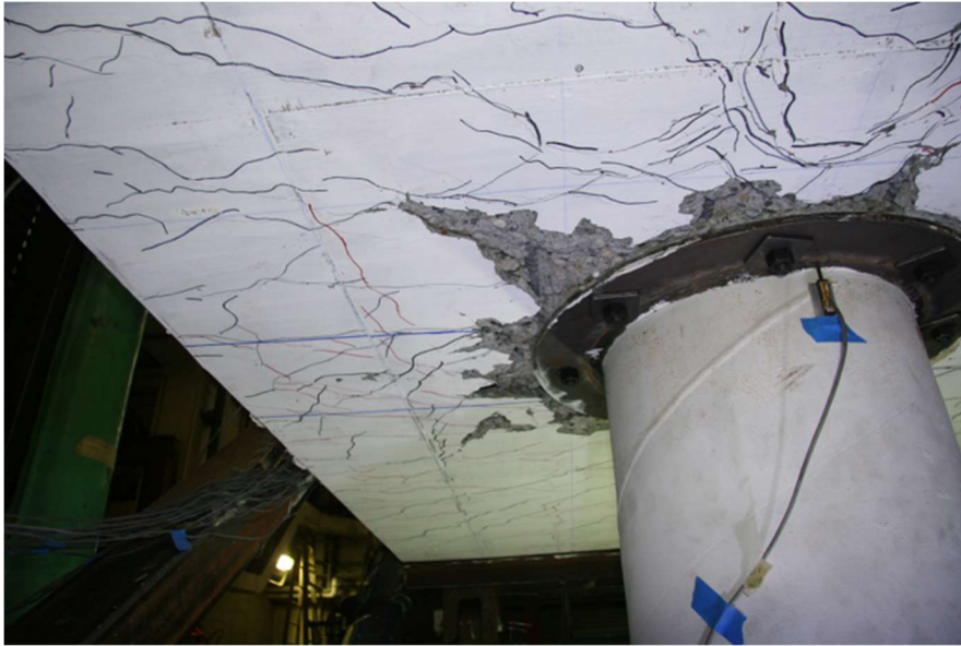
Figure 4.22. Crushing on North Side of Bottom Face – 5.63% Drift (PTB_4.5_1_0_6)
