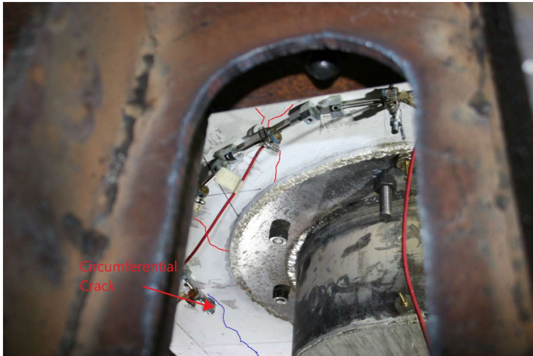
Figure 6.2. Cracking on Bottom Face of Northeast Slab – 500 kips (PTB_4.5_1_0_P)
