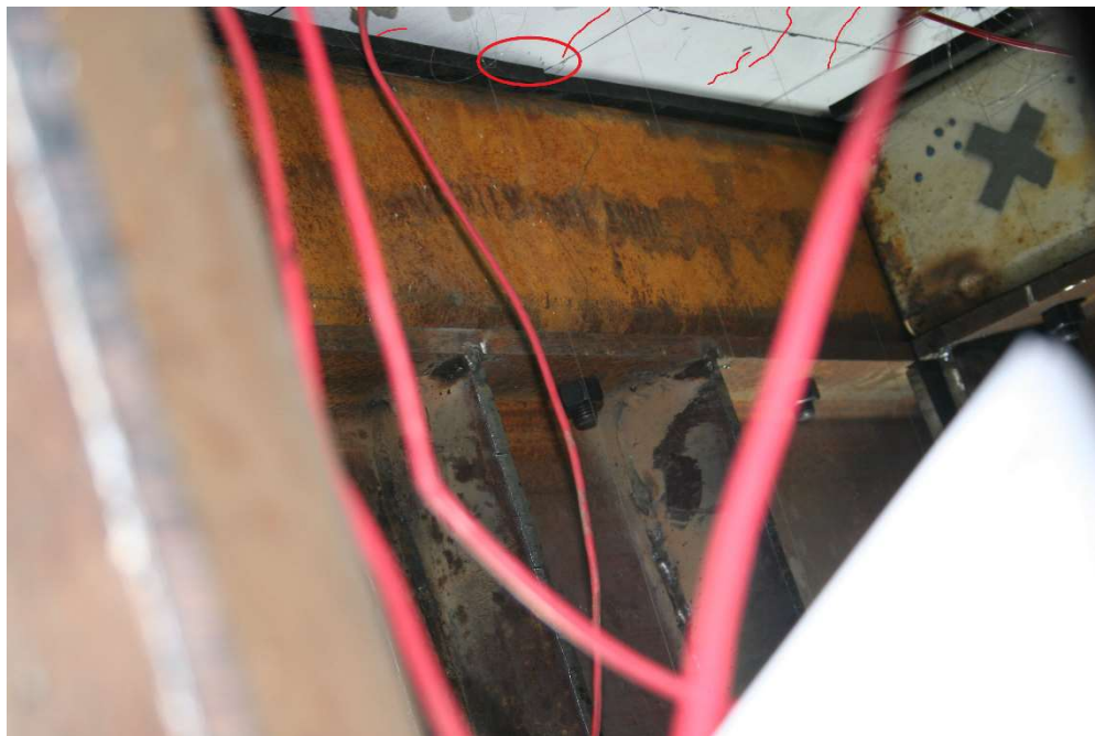
Figure 6.25. Bottom Face of Slab near North Support – 700 kips Post Peak (PTB_9_2_0_P)
