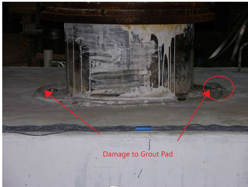
Figure 6.6. Crushing of Grout Pad North Side of Slab – 470 kips (PTB_4.5_1_0_P)
