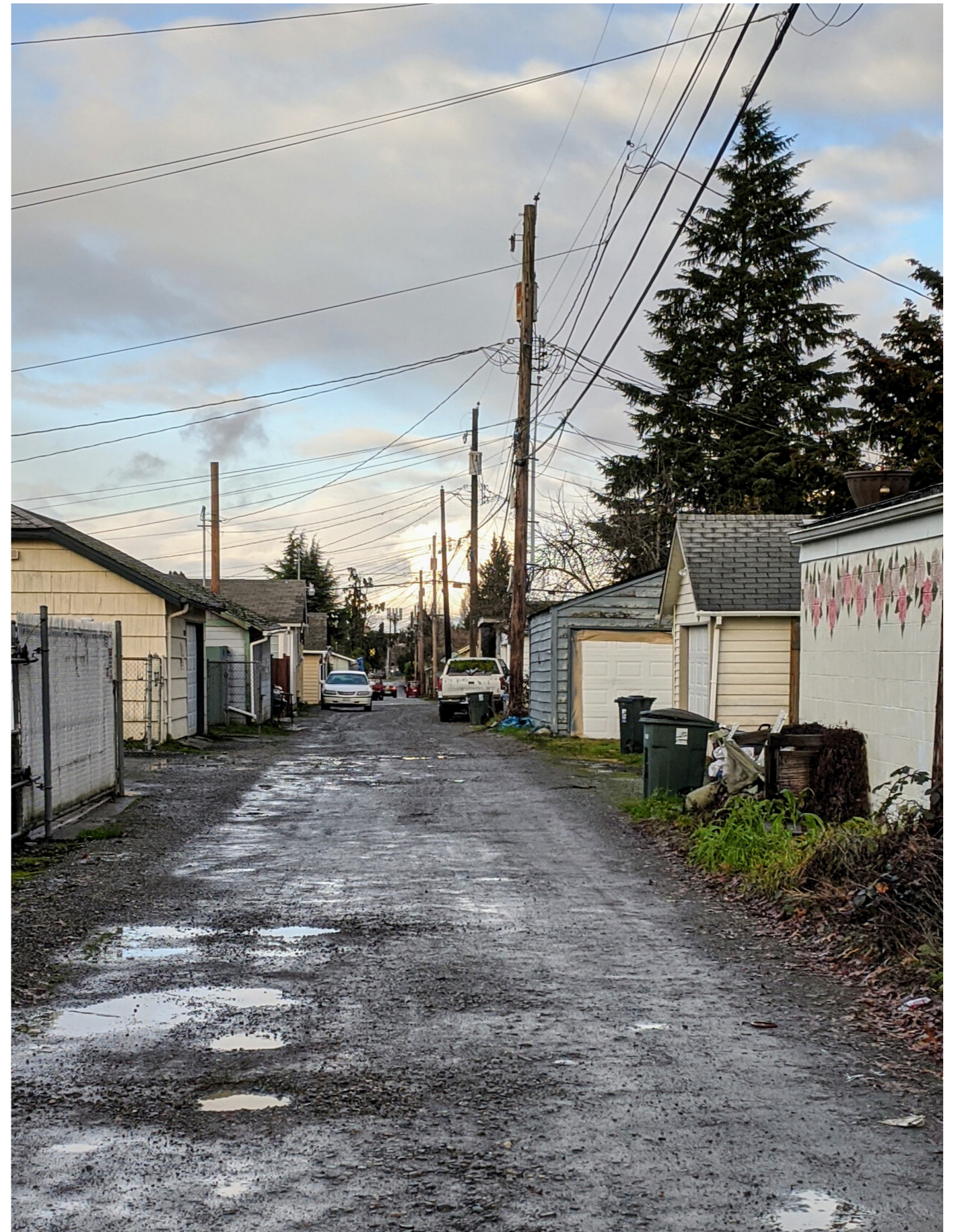
Fig. 23 Standing water in potholes along the alley between S. 43rd and S. 45th street
