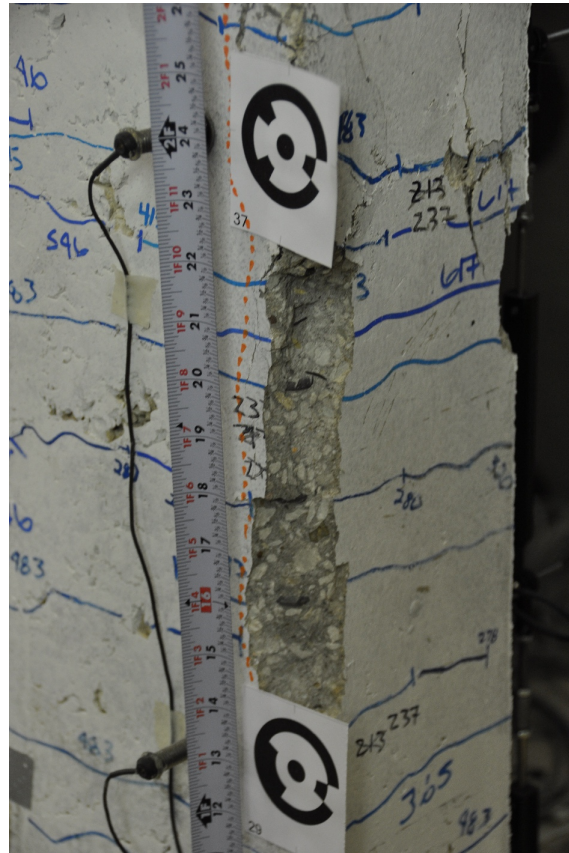
Figure 4.20: Close up of spalled region shown in Figure 4.19, tape measure referenced to base of wall
