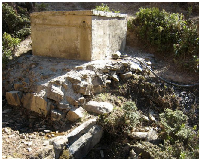
Figure 15: Pianshui Collection Tank
