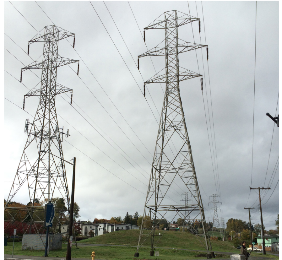
Figure 7.2: Transmission towers along S Henderson St. (Source: Author)
