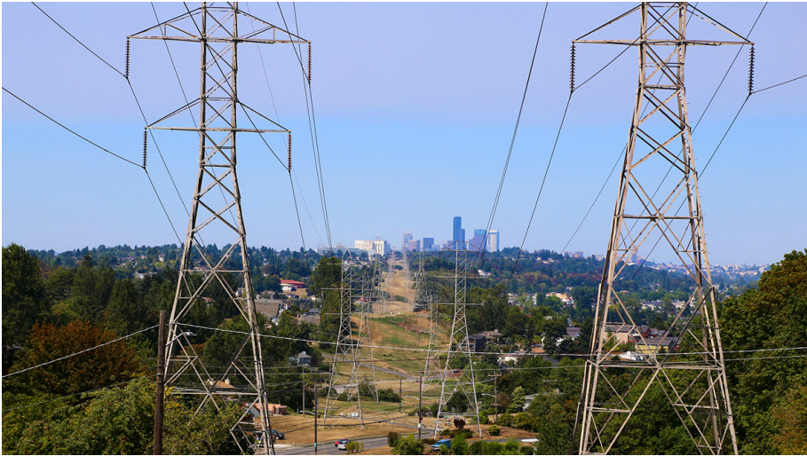
Figure 5.7: City Light Utility Corridor, looking northwest toward Downtown Seattle (Source: Seattle City Light, 2015)
