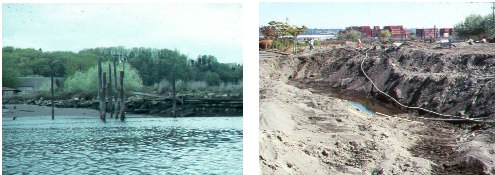
FIGURE 6. (a) T-105 site, pre-restoration, view from Duwamish Waterway; (b) view looking toward waterway during construction. Photos by C. Tanner.
