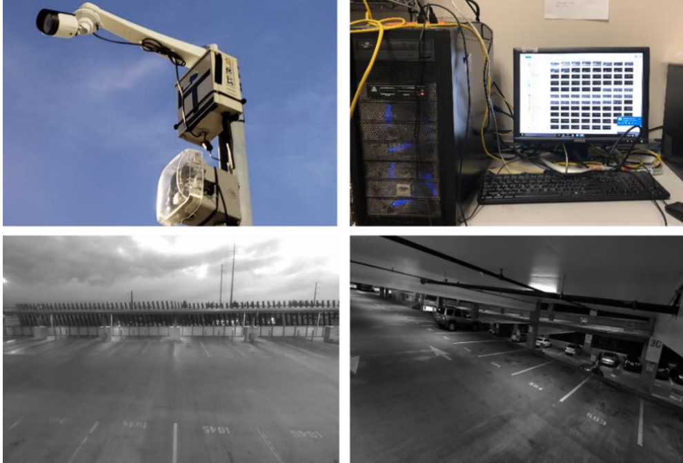
Figure 4-5 System installation at the Angle Lake parking garage (top-left) and the server set up at STAR Lab (top-right); the bottom row displays the camera views of the devices we installed on the sixth floor (bottom-left) and the third floor (bottom-right).
