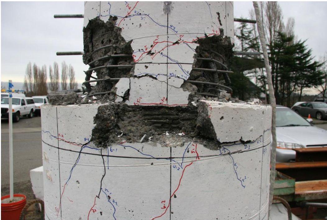
Figure C-0-6. DS-1 – Column damage after cyclic testing
