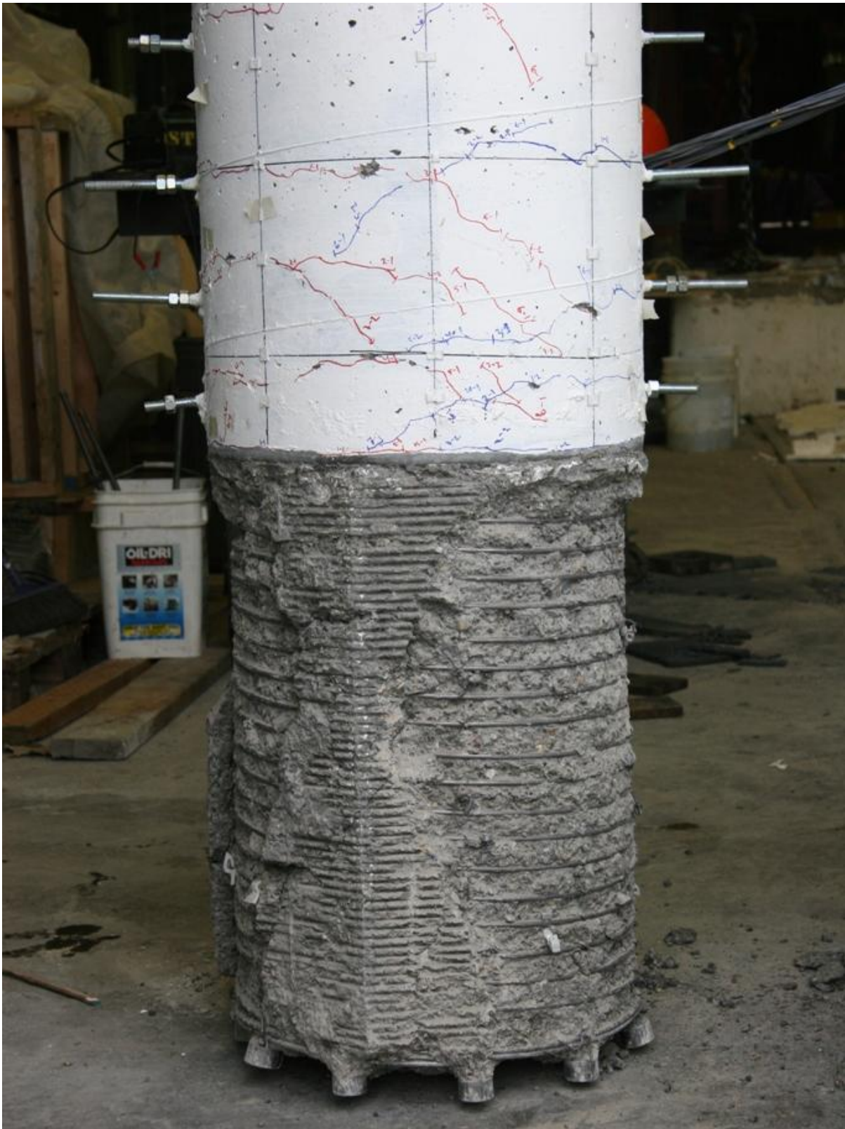
Figure C-0-13. DS-2 – Column damage after cyclic testing
