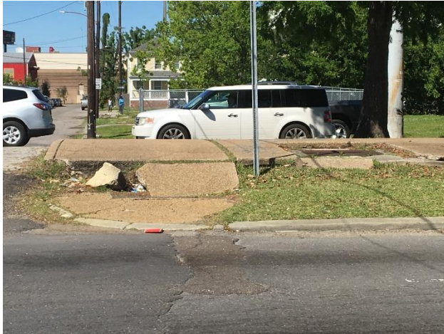
Figure IV-T Evidence of subsidence around drainage canal (17)
